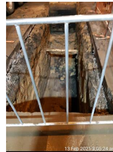
Site evidence (Elizabeth Street) – cable trench progress photographed by site staff later that night (early morning)
