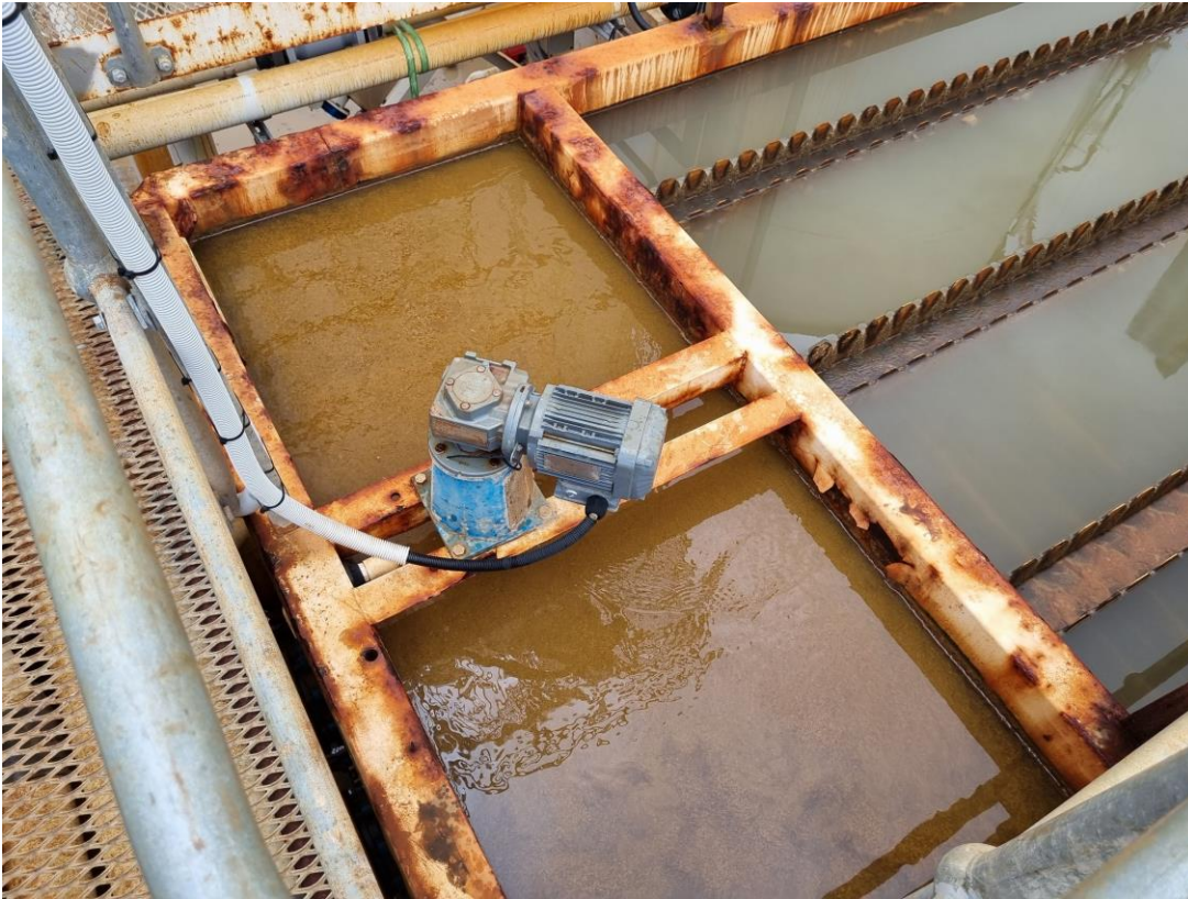
Plate 6 - Flocculation zone in WTP
