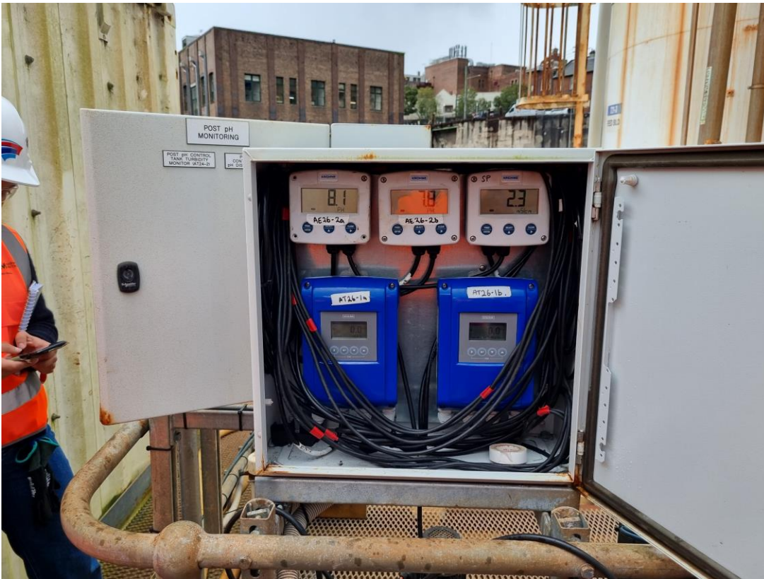
Plate 7 - In line turbidity and pH monitoring at WTP
