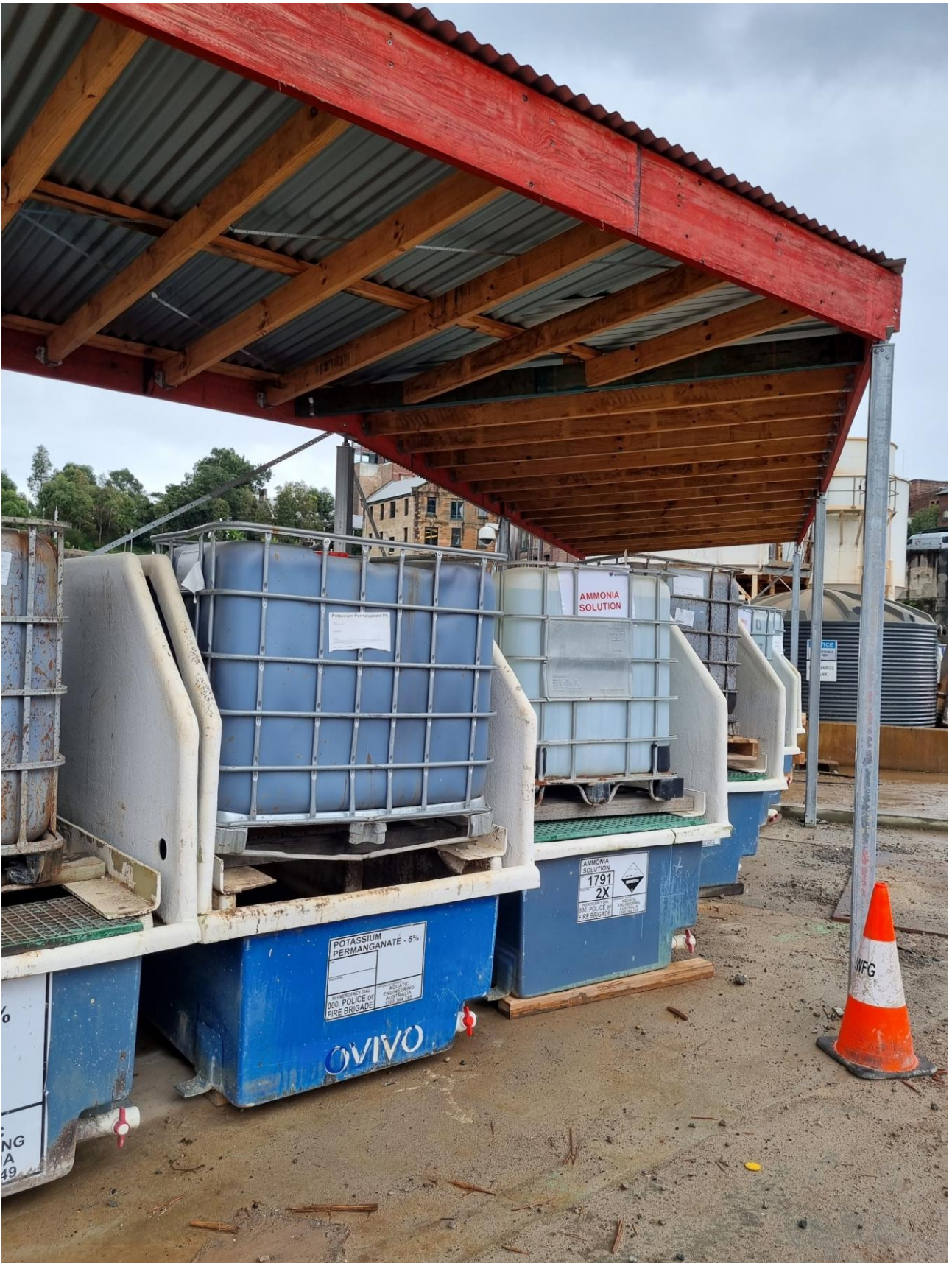
Plate 3 - Chemical storage area at WTP with roof to reduce rainfall ingress into bunded areas
