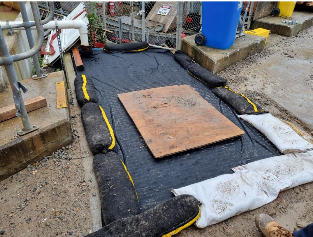
Plate 5 - Discharge outlet pit protected with geofabric and sand bags
