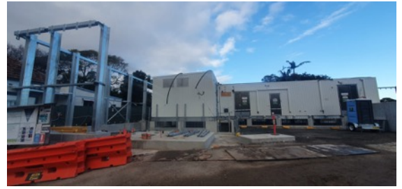
Surry Hills BPS works – Belmore St worksite: Second cable jointing works underway
