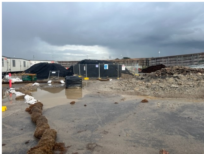
Stockpiles of hazardous waste
