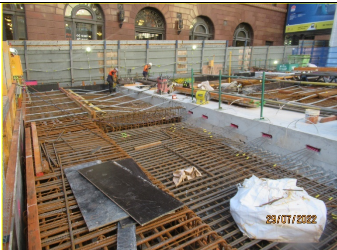
Martin Place – Construction of new slab where pedestrians will be directed to once bridge is closed.
