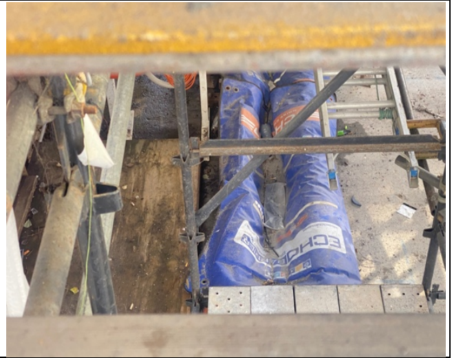
Victoria Cross North Yard Area: Observation of noise blankets in place around concrete pump lines (good practice)
