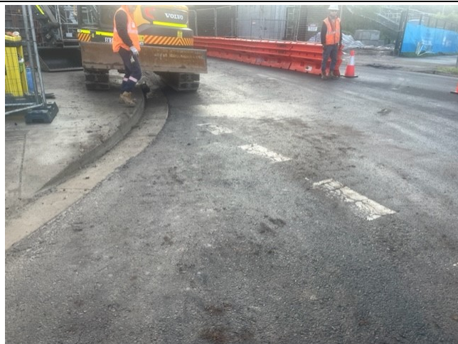
Wairoa Street Bridge, Campsie: Traffic control was in place to navigate a lane closure on Wairoa Street. Tracking to be monitored ongoing.
