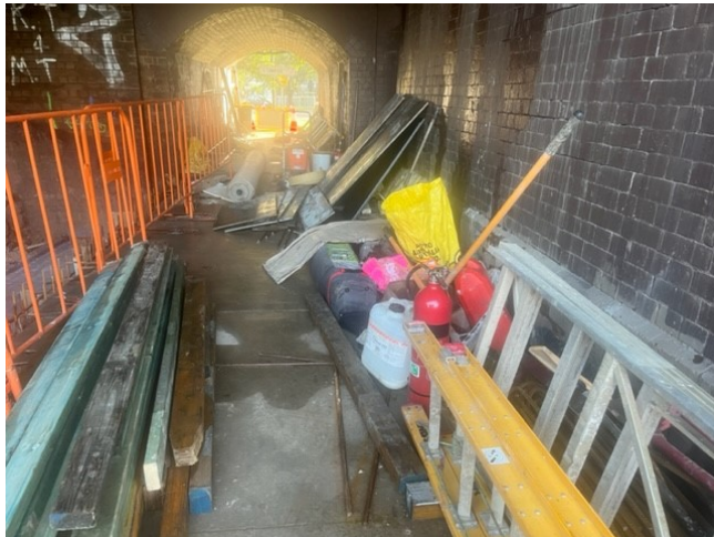
Wairoa Street Bridge, Campsie: Jerry cans of ULP were stored without secondary containment. A spill kit was not located within the near vicinity.
