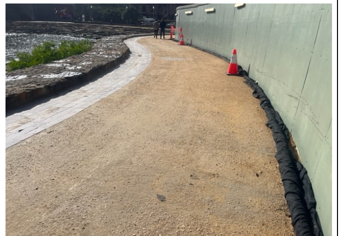
Nawi Cove foreshore after spill clean-up (incident 13/7/22)
