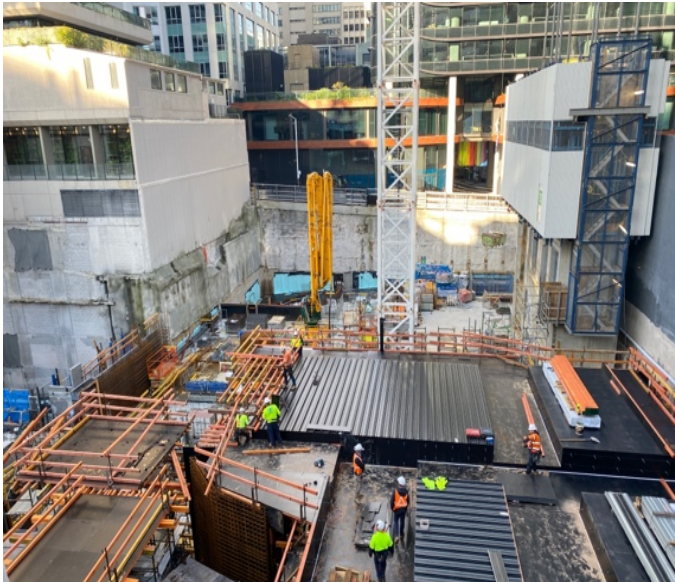
Victoria Cross South (VCS): Jump form at VCS. Steel fixing and concrete pours occurring at Level B3
