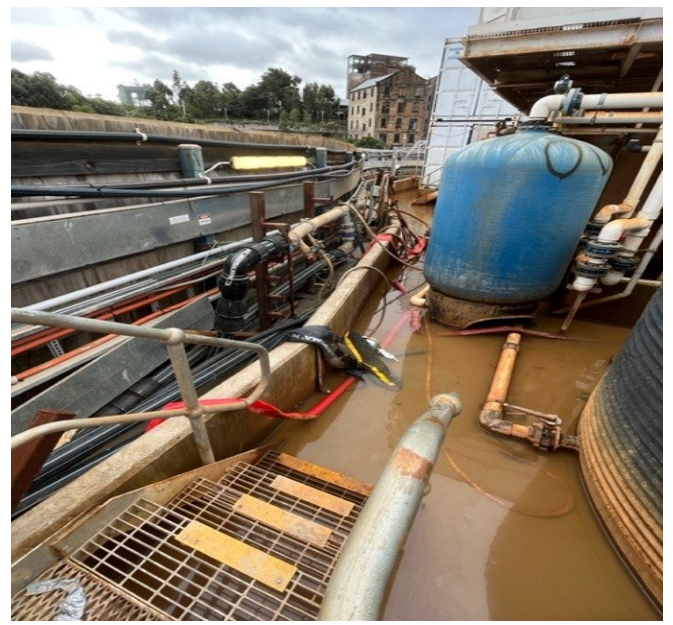
WTP bund that overflowed during incident on 13/7/22
