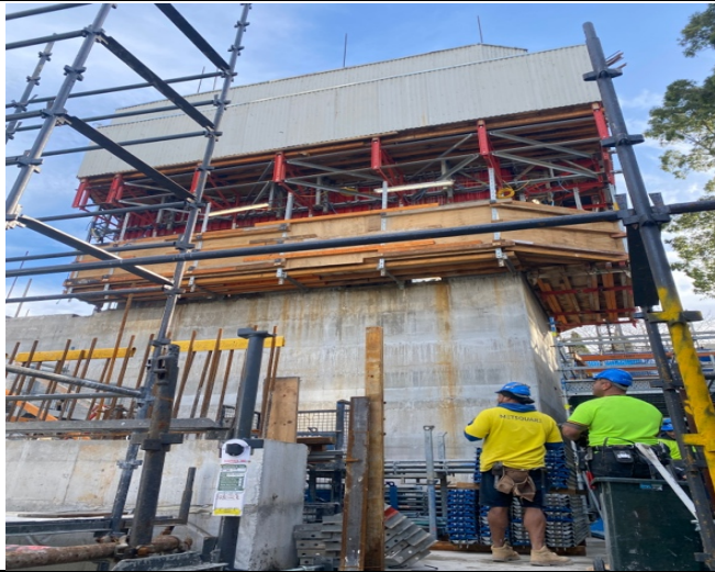
Victoria Cross North Shaft: Core jumpform noted above ground level and concreting works in progress for slab (1 floor).
