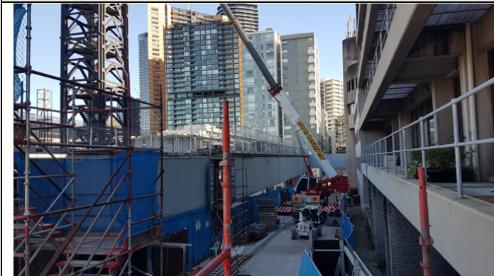
Clarke Lane North MAF – Materials Storage and Mobile crane operations in support of tower cranes
