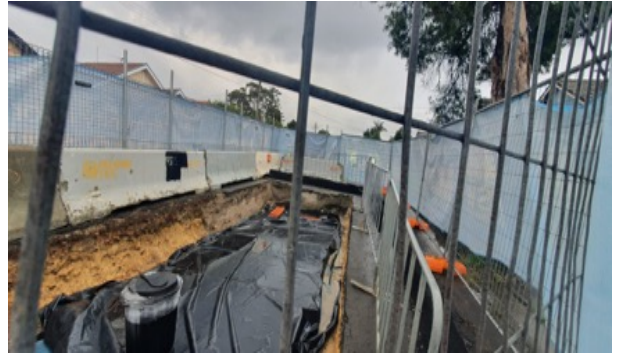
Anzac St – Joint Bay worksite (BPS works) - Anzac St Joint Bay backfilled.
