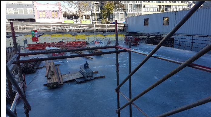
Site A view Northwest - Concrete slab poured on B/B0 girders over station atrium
