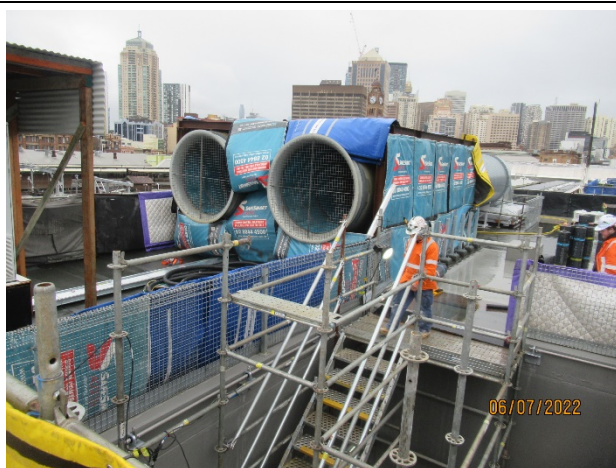
Temporary Ventilation fans on top of the ventilation building
