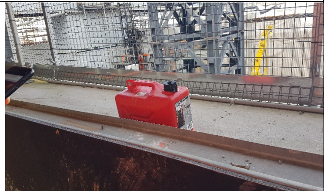
Clarke Lane North – Flammable liquid container left on capping beam inside hoarding
