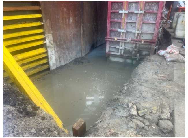
Wairoa Street Bridge, Campsie: Accumulated water transported offsite for disposal (high pH).
