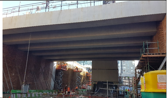
Site A view Northwest - Concrete slab poured on B/B0 girders over station atrium
