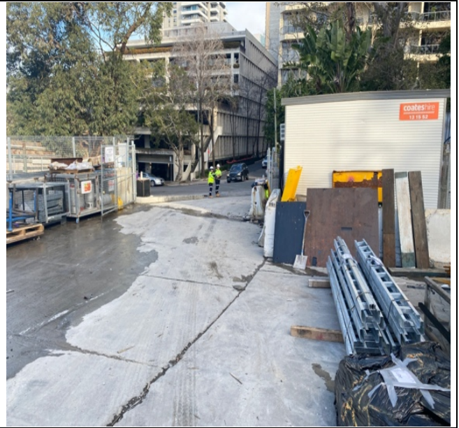
VCN -McLaren St: Site access/egress on McLaren St was observed to be generally tidy at the time of inspection
