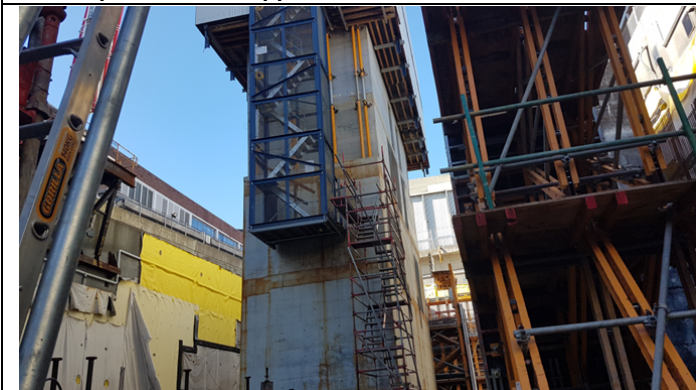
Level B2 South: Steel fixing for perimeter walls, with jump form at Level 2.
