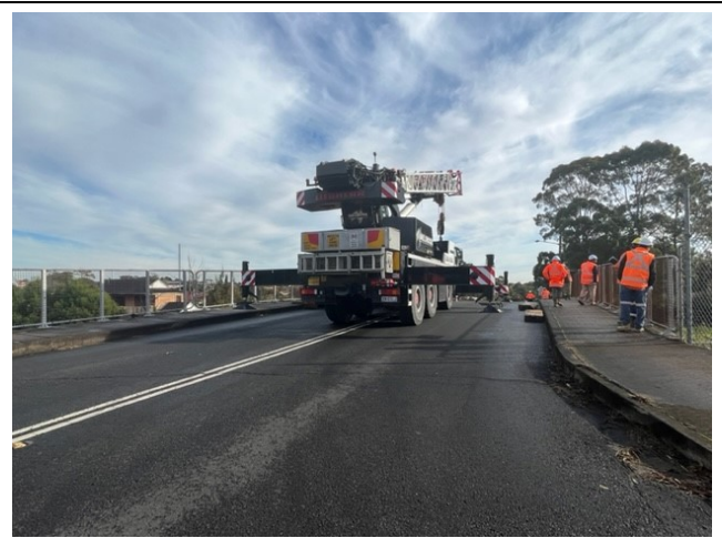
Loch Street, Belmore: Full road closure in place on Loch Street Bridge to allow crane to lift beam onto GST alignment under the bridge. A Consistency Assessment was approved for this activity.
