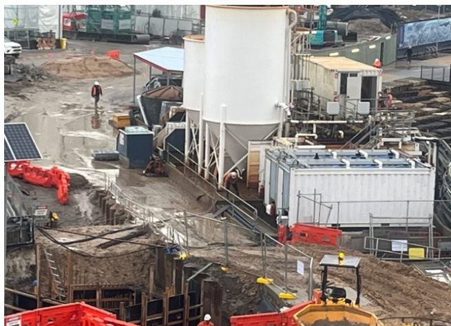
WTP bund water and sludge being emptied onto the haul road (NC with REMM WM1)
