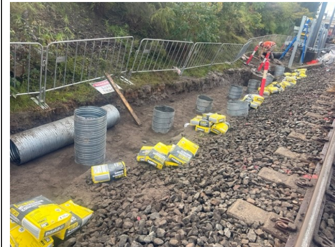
Breust Place, Punchbowl: During GST post installation an underground stormwater pipe was damaged. Temporary protection measures were established at the time of the incident to reduce the risk of sediment entry into the system.
