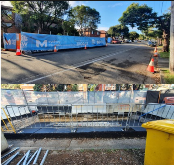
Gould Street – Joint Bay worksite (BPS works): Joint Bay remains open and dewatering during standard construction hours, as required. Bund control noted to remain in place.
