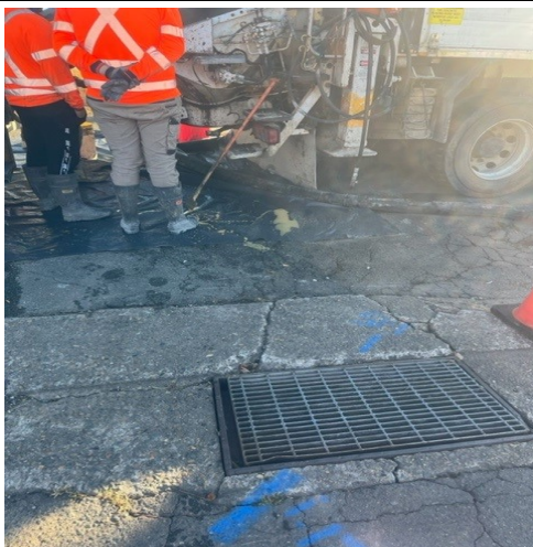
Park Street, Campsie: Cement pumping works adjacent to unprotected drain
