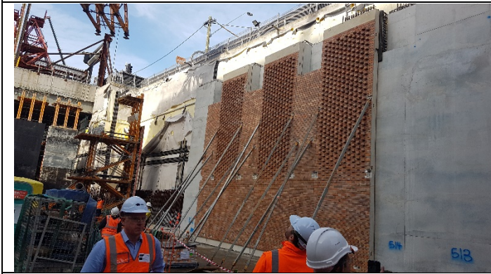
Site A view Southeast - B2 - B1 east perimeter wall with finish panels installed in sections
