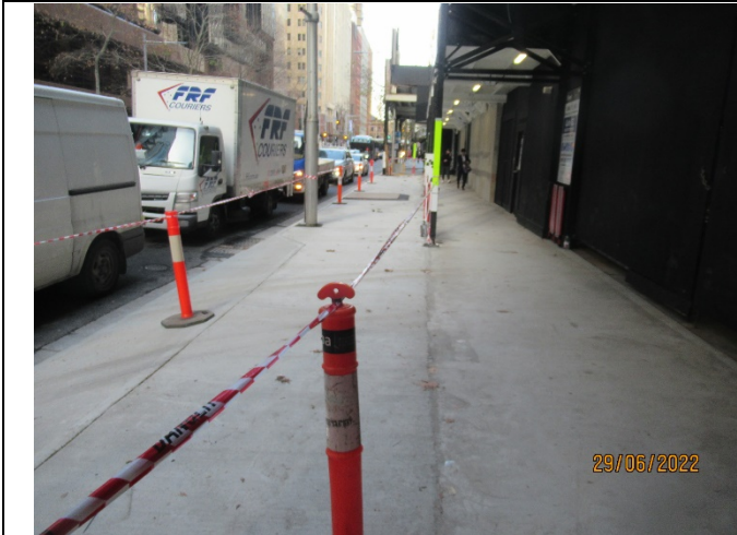
Martin Place North – new pedestrian footpath constructed adjacent Elizabeth Street to allow access to site
