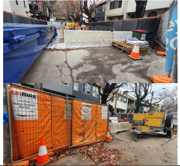
Belmore St Joint Bay: Bund and noise blankets installed around the generator.
