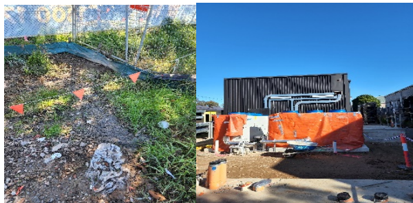
Belmore: Concrete washout adjacent to ESC, and MSB chillers
