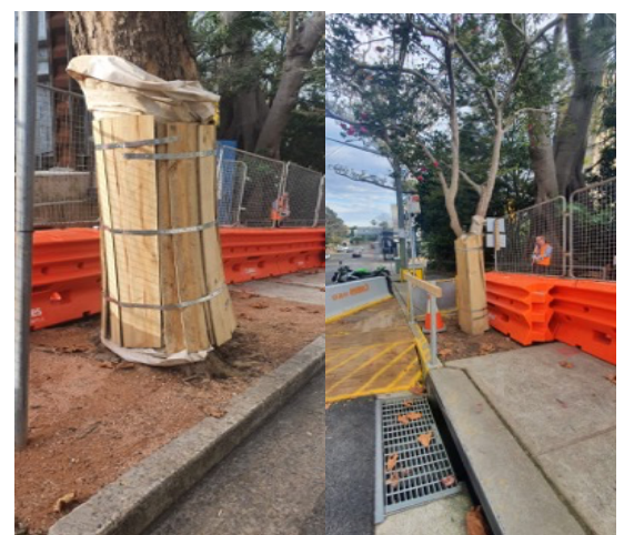
Victoria Cross North: Tree protection noted to be installed around trees, along hoarding worksite.
