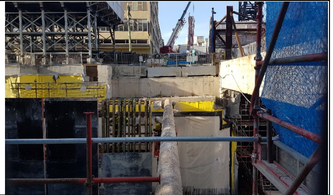
Site C view south– Clarke Lane bridge removed with capping beam remaining
