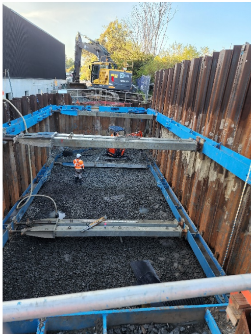
Marrickville MSB – WTP reinstated and ULX pit dewatered and backfilling with ballast.
