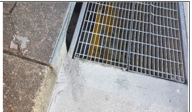
Clarke Lane South – Concrete slurry spill was evident on the eastern side of the lane
