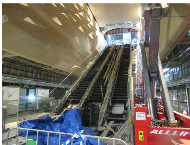
Escalator to the Metro decl level
