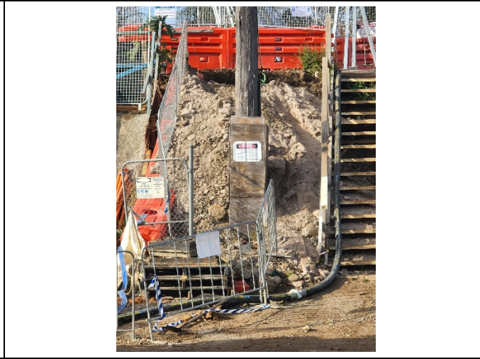
Lakemba MSB – Material stockpiled on embankment
