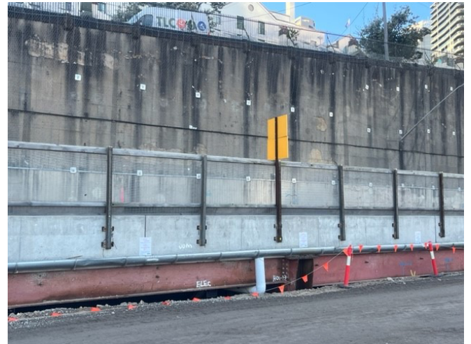
Hickson Road heritage wall – Temporary stormwater to be supported by existing rock anchors to allow Hickson Road demolition to occur
