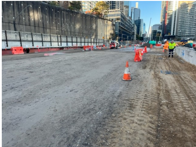
Preparation works for the temporary alignment for the Hickson Road switch were ongoing
