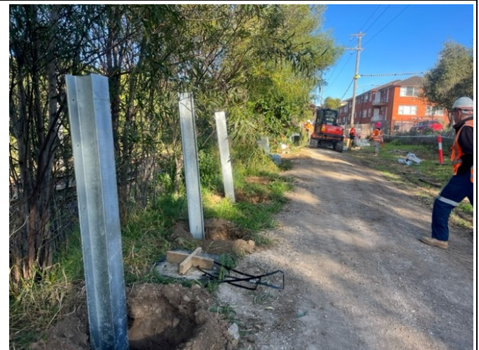
Alice Street, Wiley Park: Broken branch (raised as incident)
