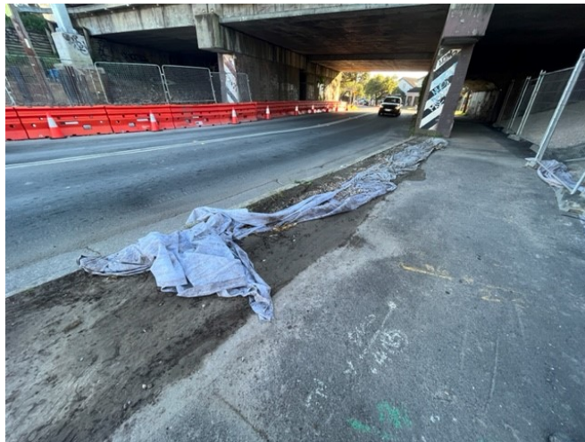
Wairoa Street Bridge, Campsie: Exposed disturbed surfaces increased the risk of dust and/or sediment runoff offsite
