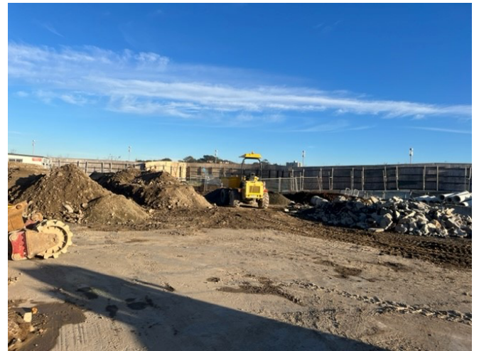
Stockpiles of hazardous waste (to be covered and controlled)
