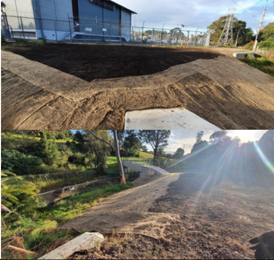
Pat O' Connor Reserve - Cable Bridge Site (Ausgrid side): Topsoil placed and jute mesh remains on batter; with hydro mulching works scheduled depending on weather.
