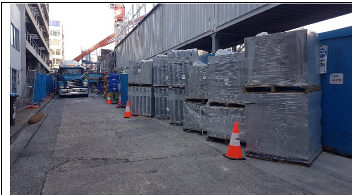
Clarke Lane North MAF – MAF beyond the approved limits, and materials are not stored in accordance with REMM LV1
