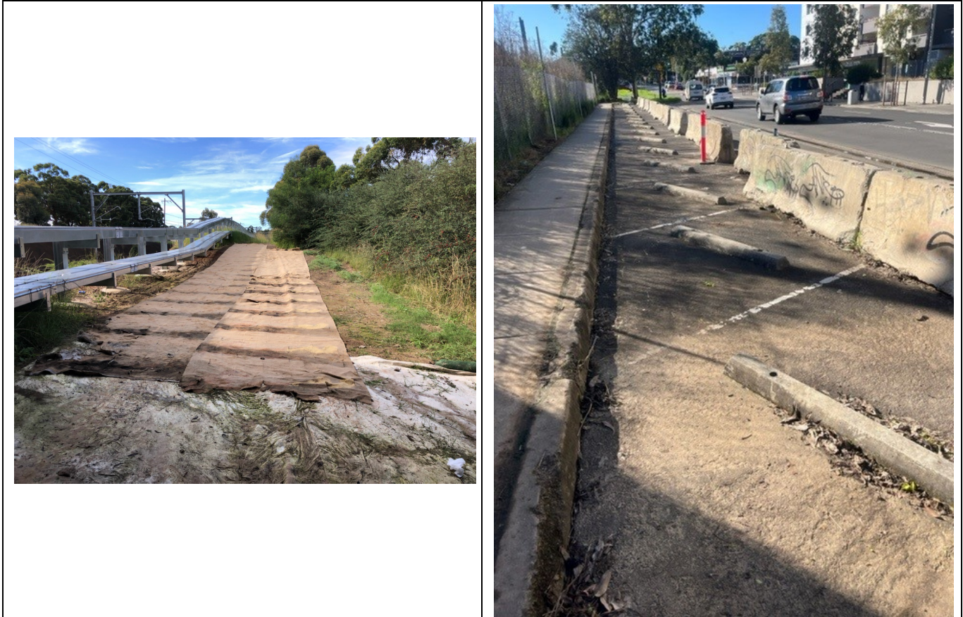
Stabilisation of a former work area with jute mat and seed, Stacey Street Bankstown
