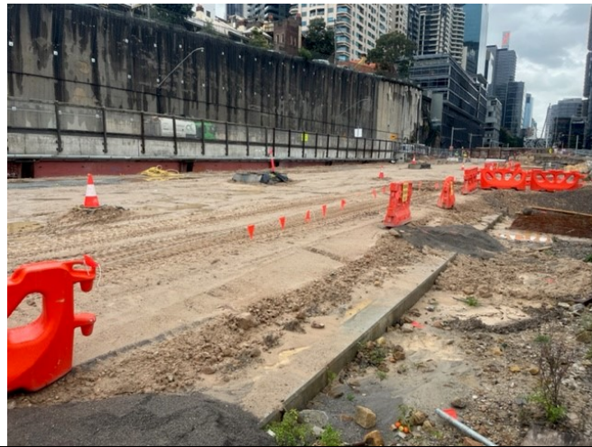
Backfilling and service installation on the roof of the station box was ongoing, in preparation for the Hickson Road switch
