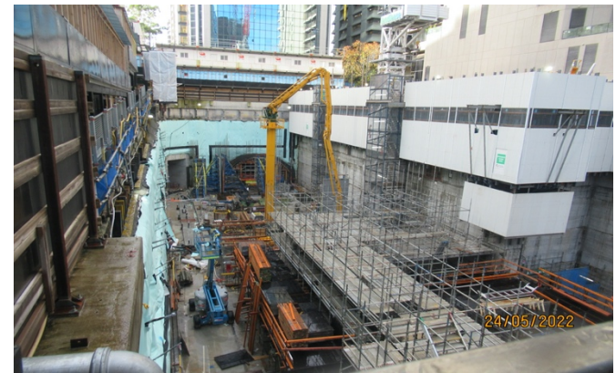
Victoria Cross South – Station Entry: Jump form and general FRP operations ongoing.
