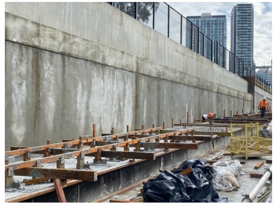
Northern connection: Final track slab form can be seen to the rear right of this image.
