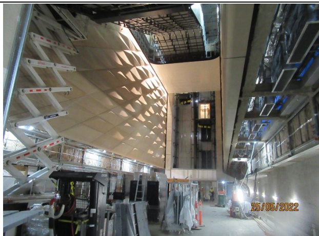
Lifts to the Metro decl level
