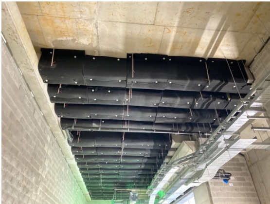
Southern Dive - This image shows acoustic insulation installed to the roof of one of the levels of the M&E building.
