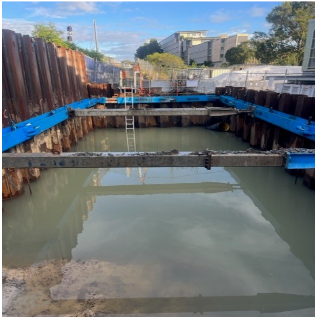
Marrickville MSB – Accumulated water in the ULX pit and WTP removed
