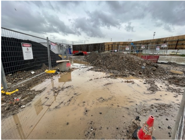
Covered hazardous waste stockpile (left) and GSW (right)
