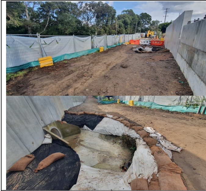
Canterbury TSS: ESC noted to be installed along sections of the site and general housekeeping in this area was observed to be good (positive observation).
