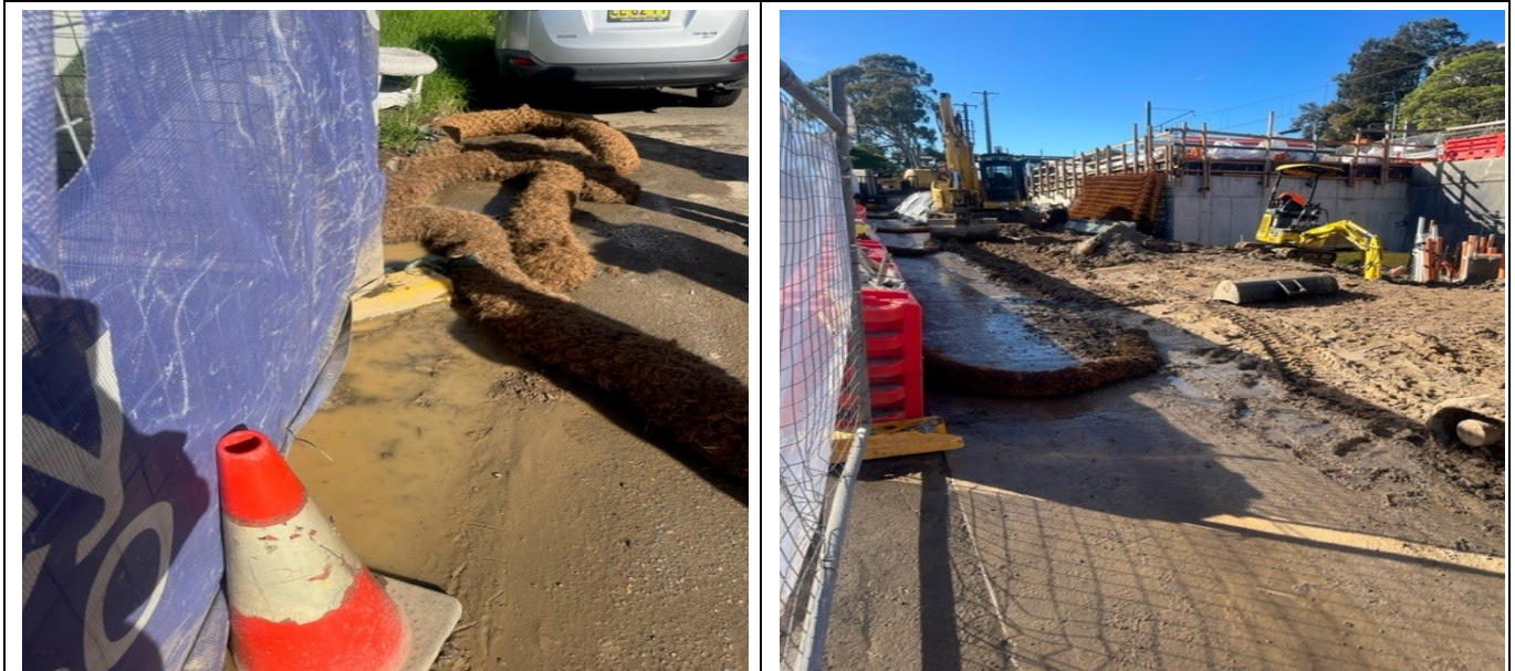
Lakemba MSB – Construction ongoing and controls in place for the continuous stream of muddy water from the site
