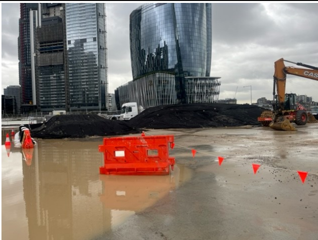
Covered tunnel spoil from Rozelle and flooding across the site
