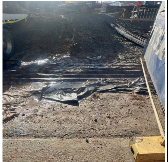
Canterbury MSB – muddy site access and tracking observed during spoil load-out
