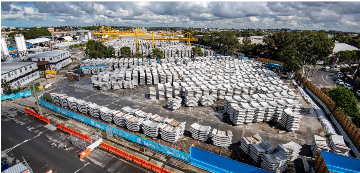
Figure 4-2 Photo of the tunnel segment storage area at Marrickville for the Sydney Metro City & Southwest project (indicative example of the proposed facility within Western Sydney International)
