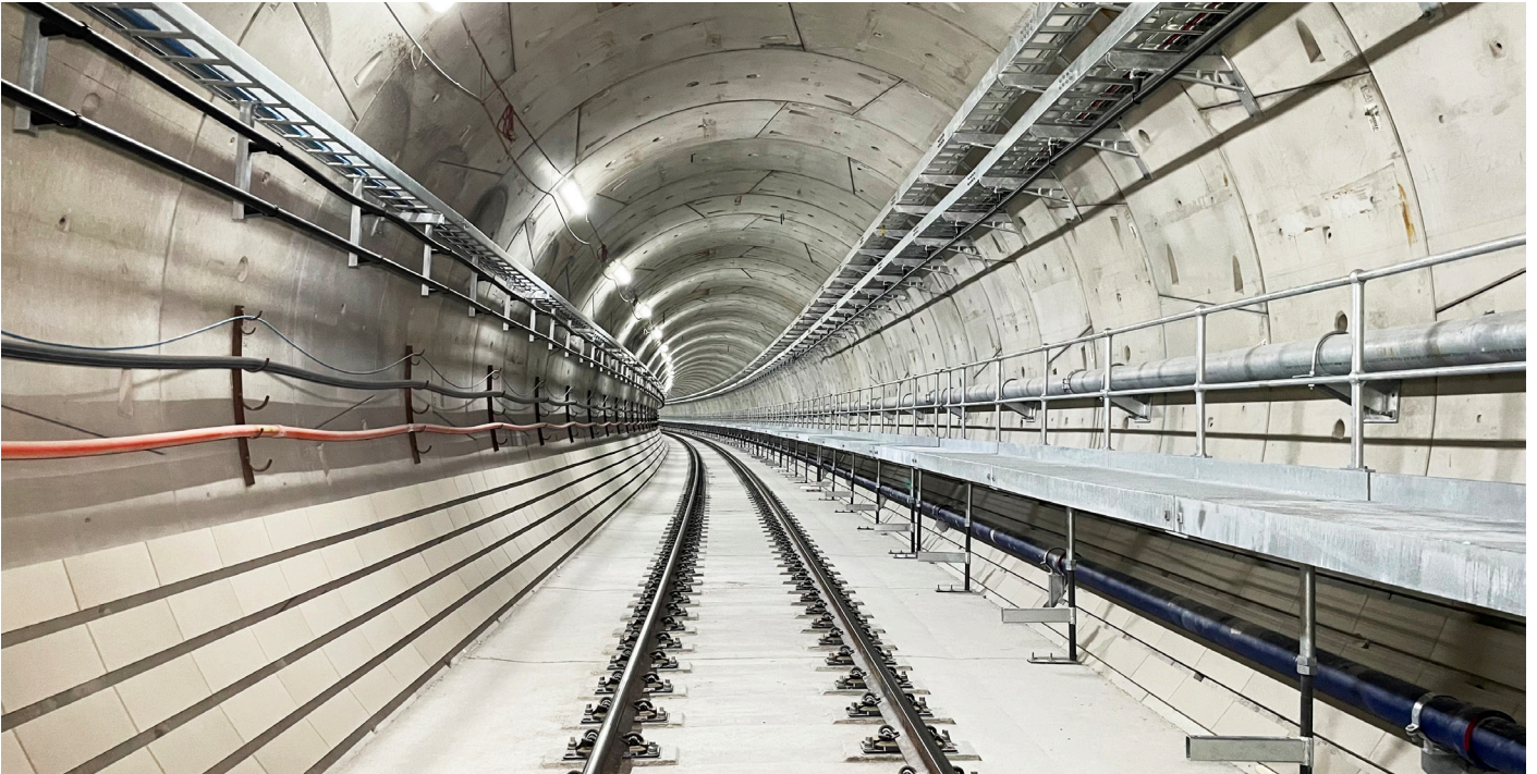
Mechanical and electrical fit-out of the twin 15.5kms rail tunnels between Marrickville and Chatswood is on schedule for completion late this year.
