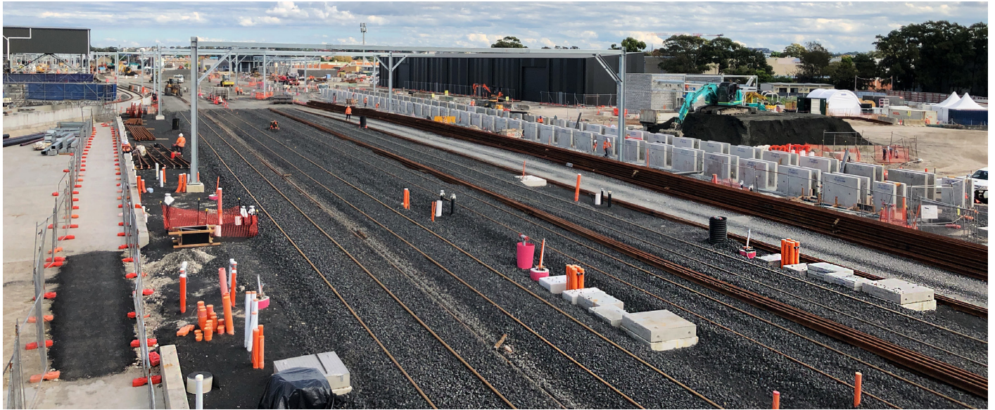
A stabling yard with enough tracks to park up to 16 metro trains is under construction at the Sydney Metro Trains Facility South in Marrickville.
