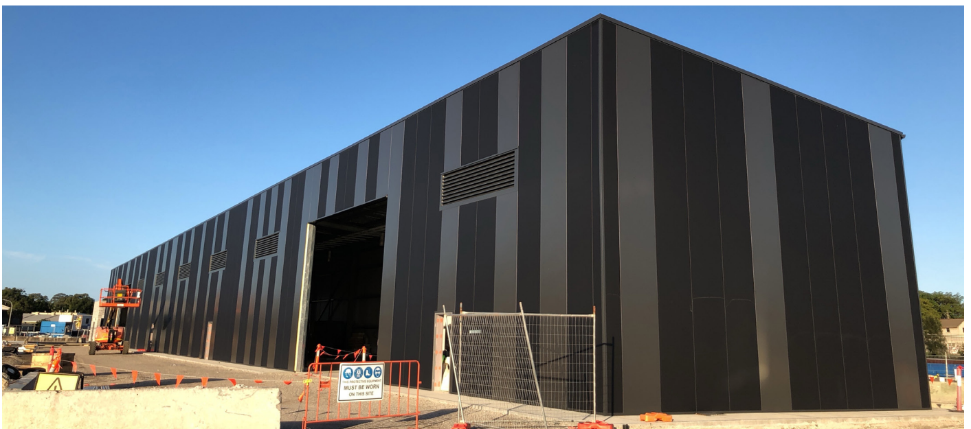
The covered store building at Marrickville has been completed, providing welcome shelter from the recent heavy rains.
