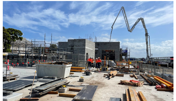
This services building at the southern dive will provide power, ventilation, communications and other services to the tunnels below.
