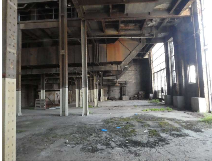
Figure 12: View of the north east corner of the Boiler House showing accessible areas for grouting equipment
