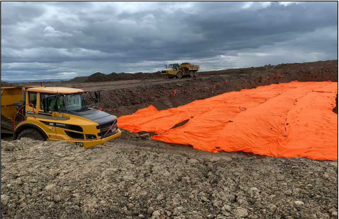
Photograph 1. Asbestos containment cell following the application of the geotextile marker layer (as supplied by the client).
