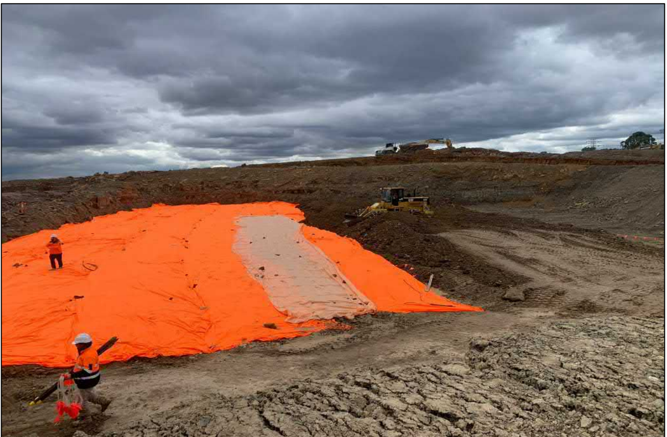
Photograph 2. Asbestos containment cell during the application of the existing site material situated above the marker layer (as supplied by the client).
