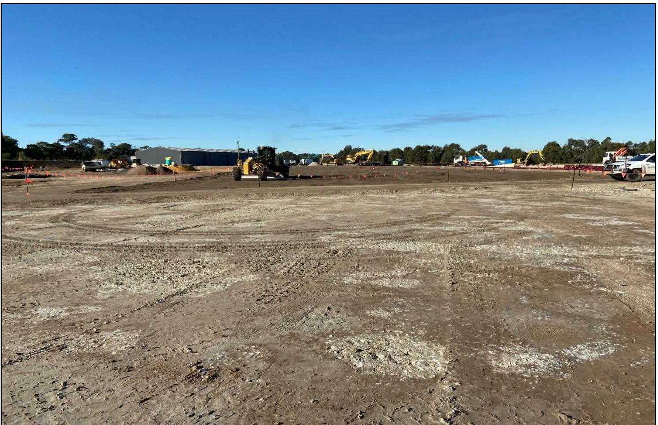
Photograph 4. Asbestos containment cell following the application of the sub-grade layer (as supplied by the client).
