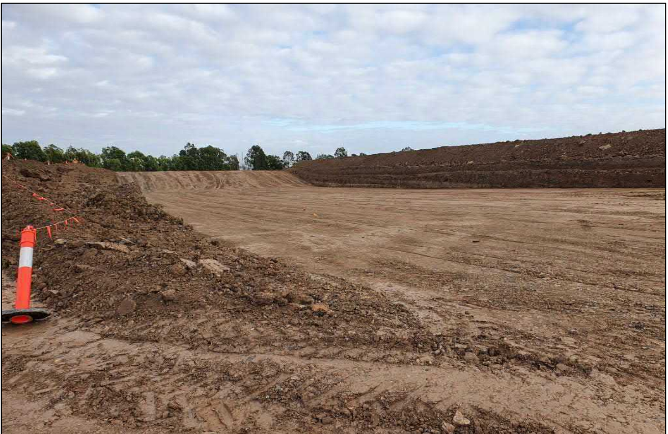
Photograph 2. Asbestos containment cell following the relocation of the asbestos-contaminated material (as supplied by the client).
