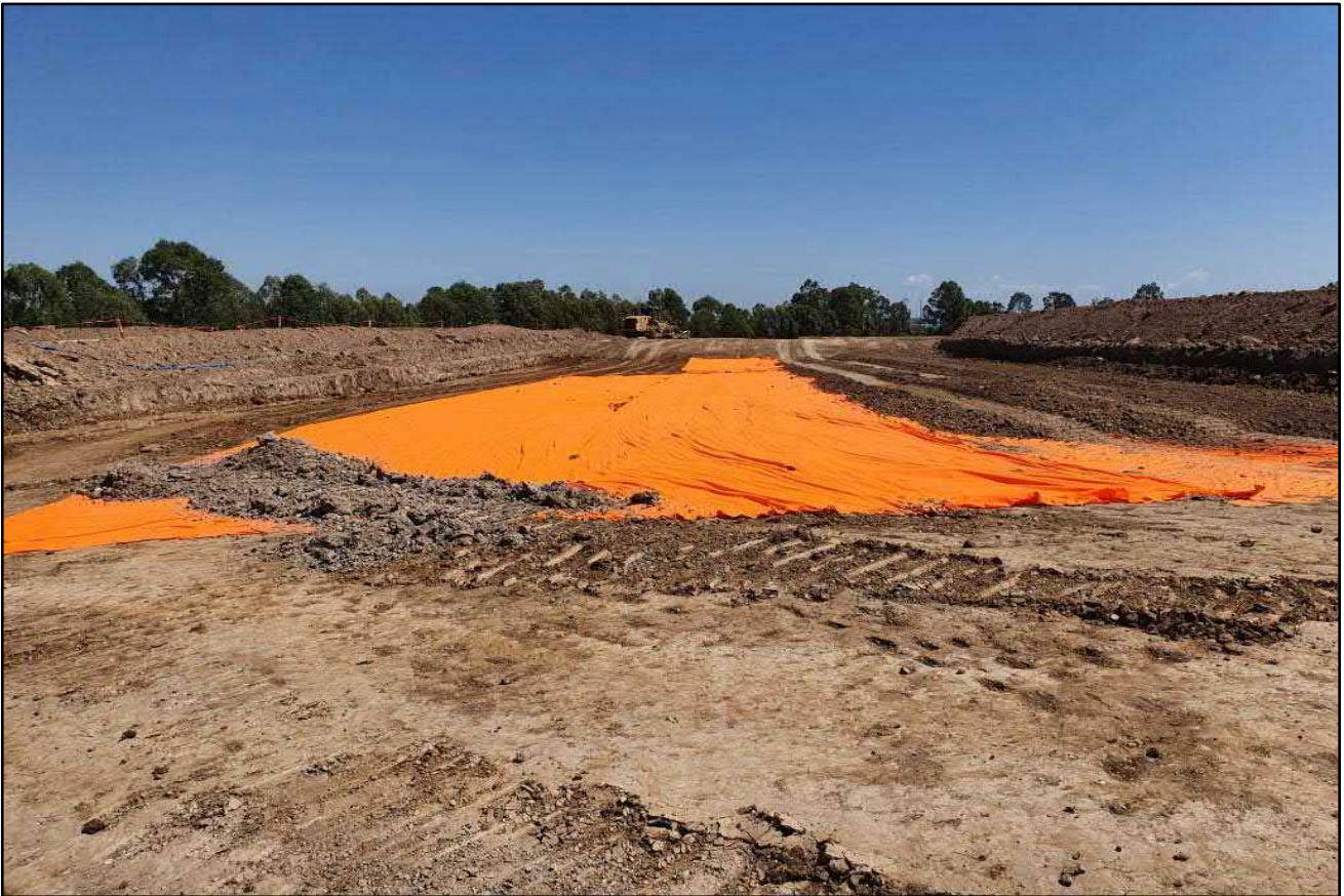
Photograph 3. Asbestos containment cell following application of the geotextile marker layer (as supplied by the client).
