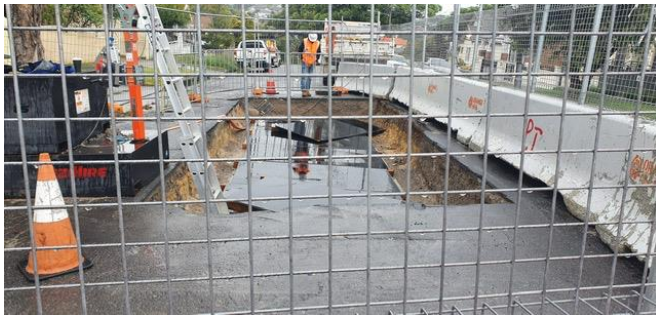
Joint Bay (JB) worksite - Anzac St - observed to be tidy. Dewatering works as required, during Standard Construction Hours.
