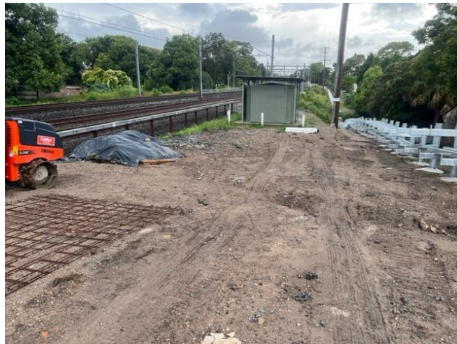
Disturbed land, Melford Street, Hurlstone Park (ERSED issues identified for rectification)
