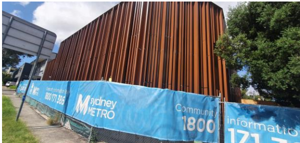
Artarmon TSS - Whiting St - Installation of facade panels on TSS largely completed (Whiting St).
