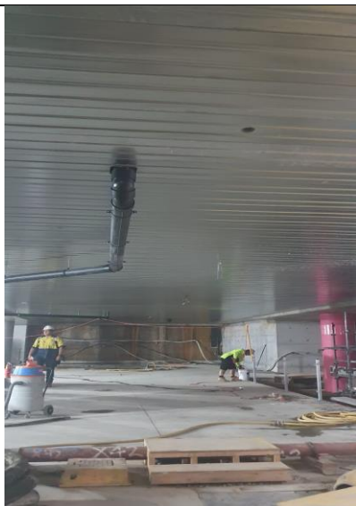
Victoria Cross South - Bondek® formwork under B4. Use of Bondek® removes need for stripping formwork.
