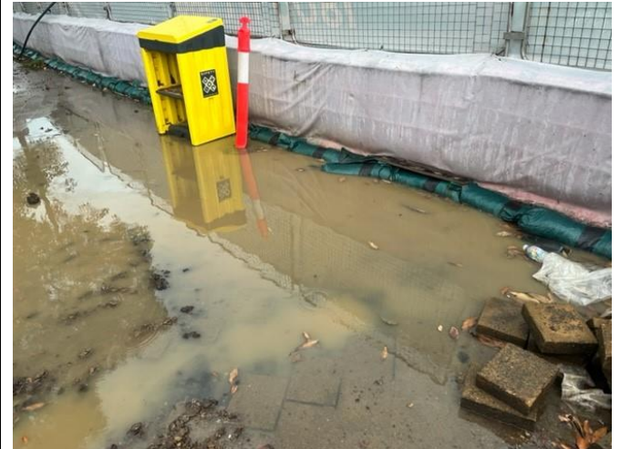
Boundary controls were at risk of overtopping during intense rainfall event at the BEW MSB Site
