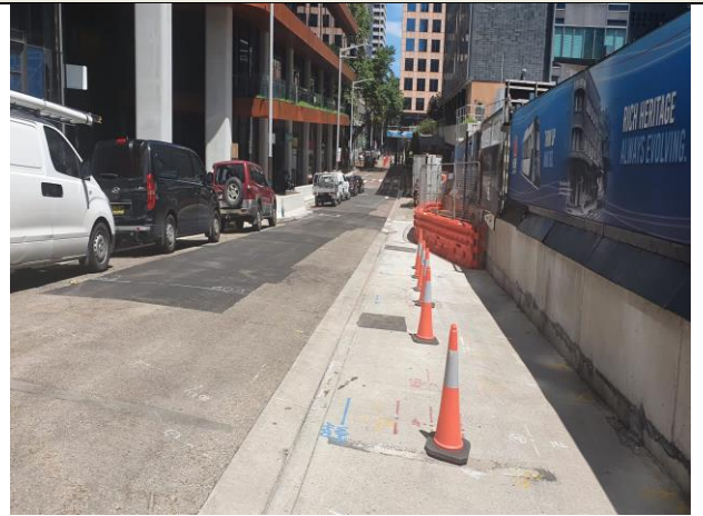
Denison Street - Stormwater works – Stage 3 area: works completed and worksite demobilised. Final connection to shaft is scheduled to occur in approximately 2-3 months.
