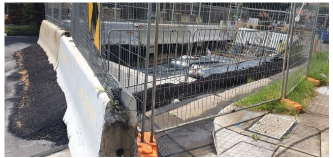
Joint Bay (JB) worksite -Cooks Ave - bund remains in place around worksite (good control), preventing water from entering SC's worksite.
