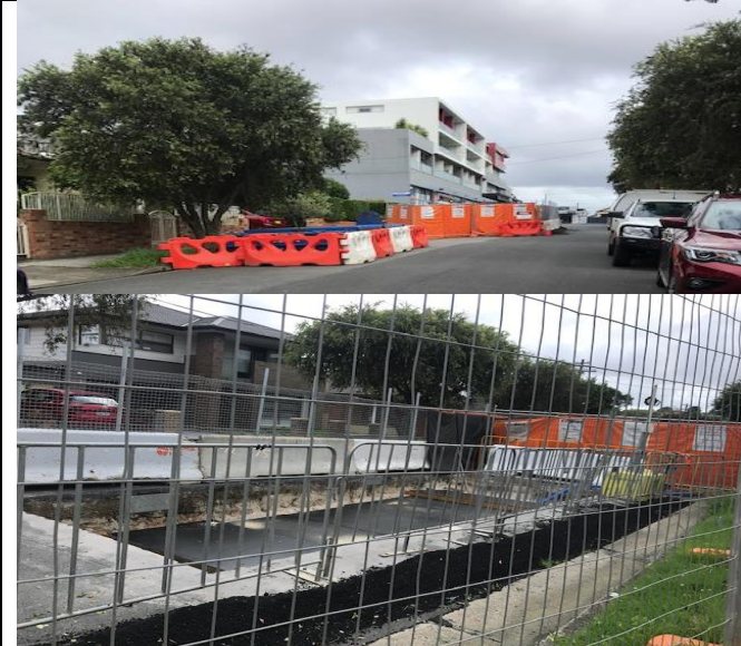
Cooks Ave– Joint Bay worksite: Noise control barriers and bund in place around worksite (good control), preventing water from entering SC’s worksite
