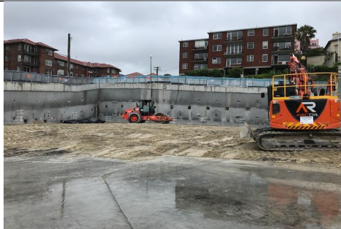
Blues Point Access Site: Placement of fill underway to restore the surface level of the worksite.
