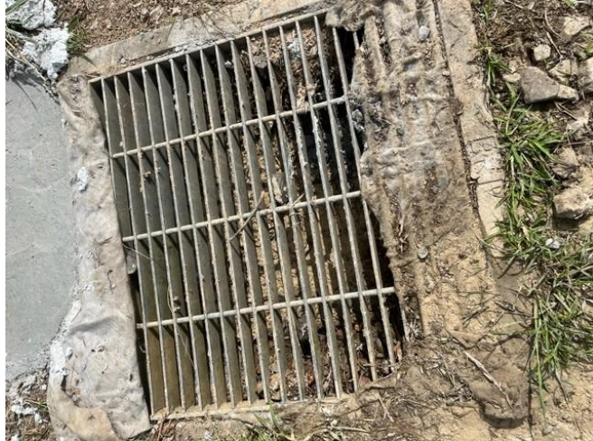
Moreton Street, Lakemba/ Belmore: Drainage grates requiring maintenance.
