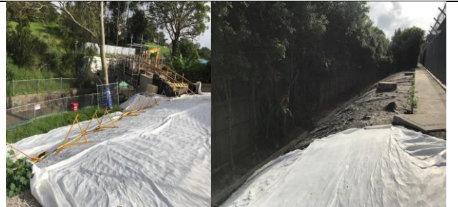
Pat O’Connor Reserve - Cable bridge worksite (Ausgrid side) – Batters remain covered and noted to have held up well, over the Christmas shutdown period.
