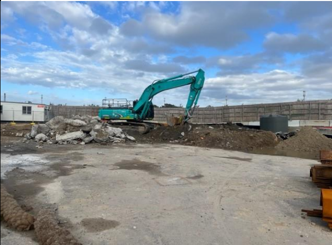
Excavation of the stormwater trench at the western end of the site was on hold pending redesign for a solution to manage water ingress.
