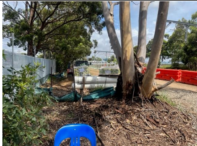
Stacey Street ULX, City-side (Gate PB15): Pipes and bags of cement were stored under the dripline of trees.
