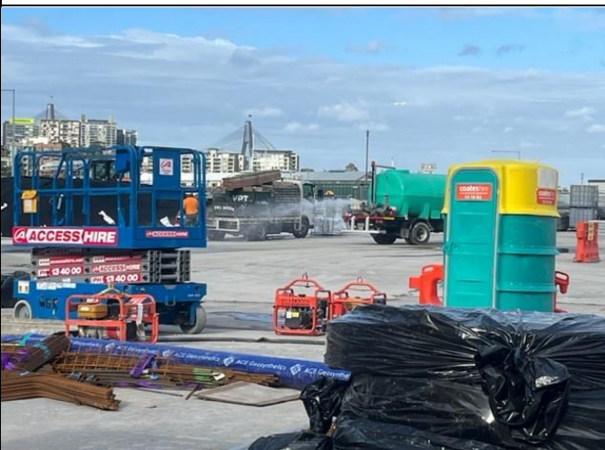
A water cart was in use to reduce impacts from a fine layer of bulldust across the site. BESIX Watpac advised a street sweeper was also in use as required.
