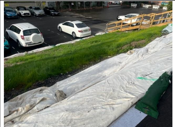
Canterbury compound: The slope from the main compound area to the lower carpark had been stabilised with grass, geofabric and sandbags at the base.
