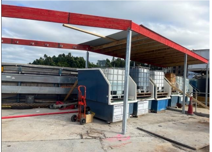
Roofed storage for IBCs containing water treatment chemicals was almost complete. Compliant storage and labelling improvements were also underway.
