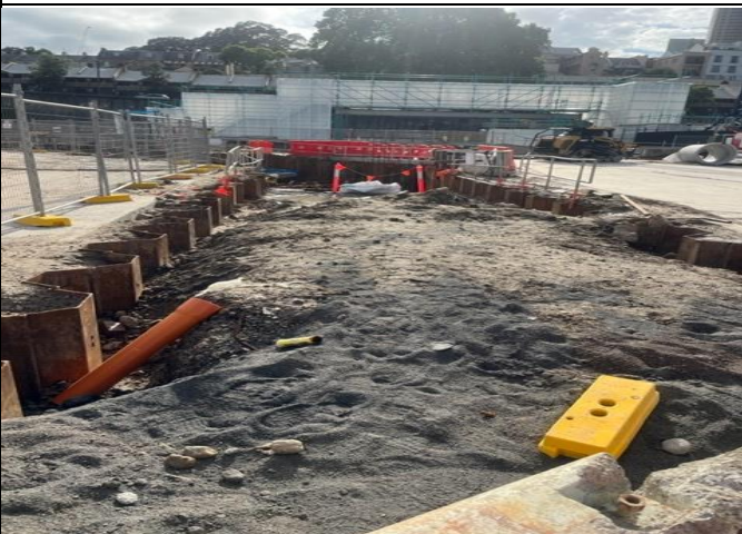
Backfill of the stormwater trench in the centre of the site. Pipe and pit complete.
