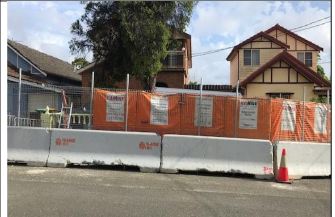
Anzac St – Joint Bay worksite: Noise control barriers in place. Compressor within trailer and generator were operating at time of inspection.
