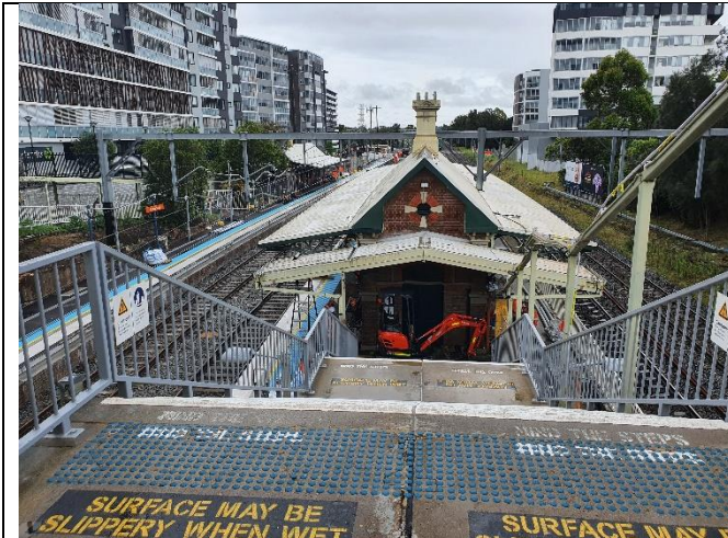
Canterbury Platform 0/1 service installation 05/01/22
