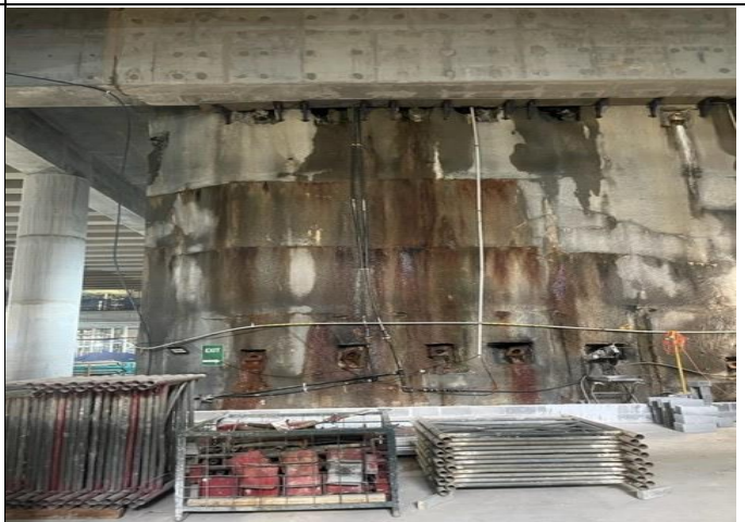
Groundwater seepage from the unsealed wall of the station box – future Aqualand development area
