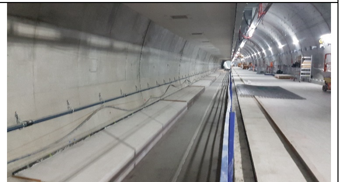
Western cavern track slab and platform with OTE above
