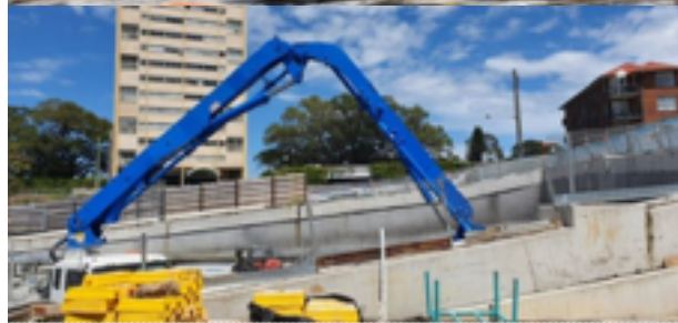
Blues Point Access Site - Acoustic shed demolition completed and erected scaffolding removed from site
