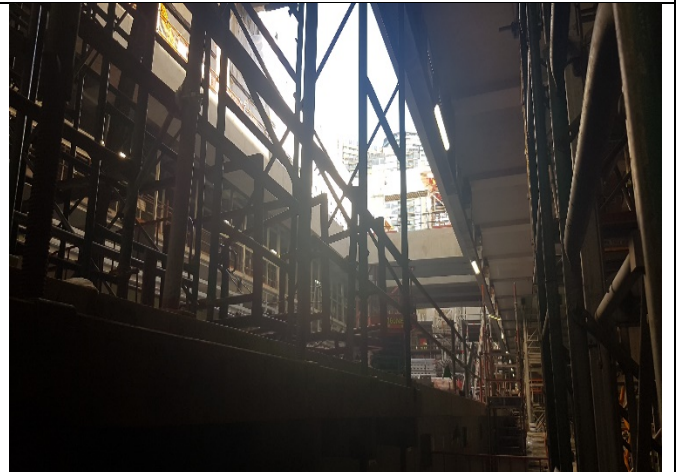
VCN - North Yard Area: No concrete pours in yard at time of inspection.
