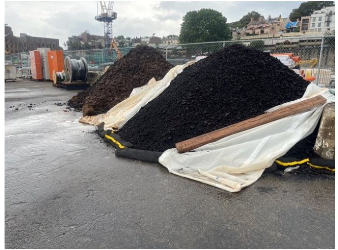
Stockpiles of filter cake were not covered prior to the Christmas Shutdown
