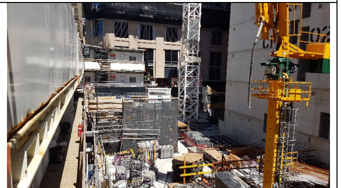
PSN western side: FRP at levels B01M and Ground
