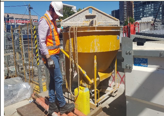
Concrete hopper that was washed out, resulting in run-off to Clarke Lane stormwater system - incident reported
