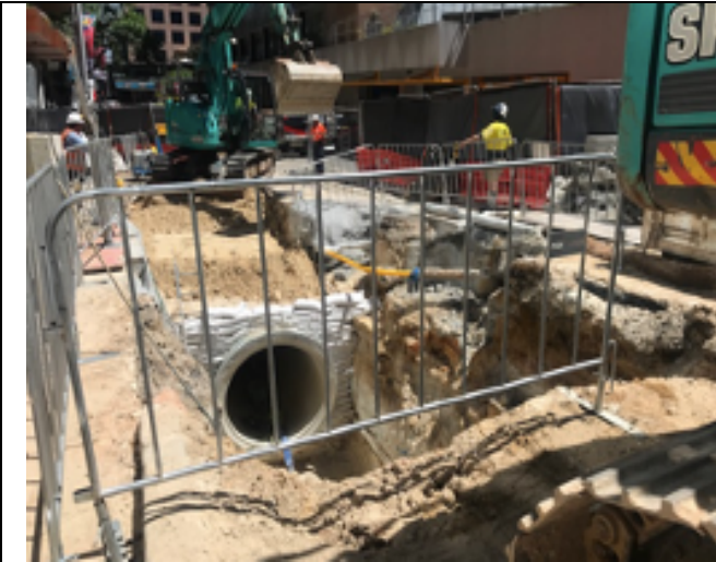
Denison Street Stormwater works – Stage 3 area: Drainage excavation works underway. Noise blankets observed in place.
