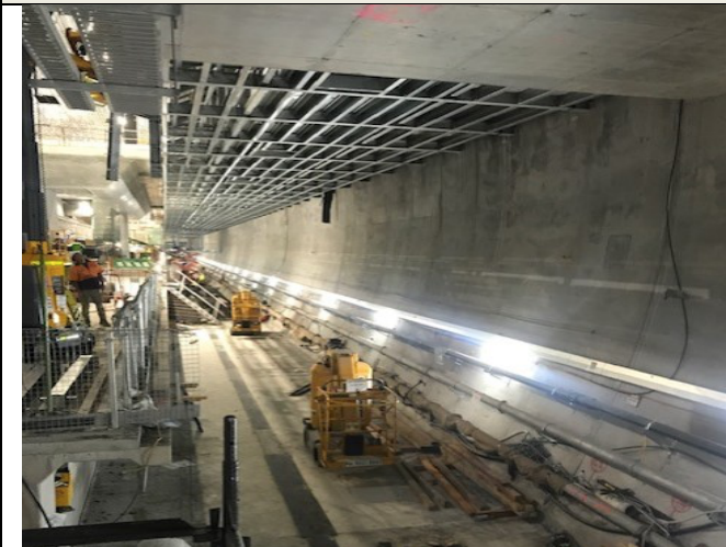
Cavern: trackway steel fixing underway on eastern side, with concrete pour scheduled to follow.
