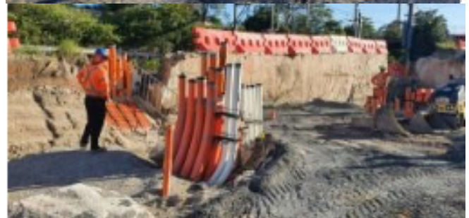
Canterbury TSS – Combined service route (CSR) works – excavation, conduit installation and backfilling continuing.
