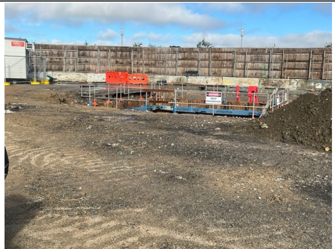
The management of infiltration of water into deep excavations associated with stormwater trunk relocation works is under discussion
