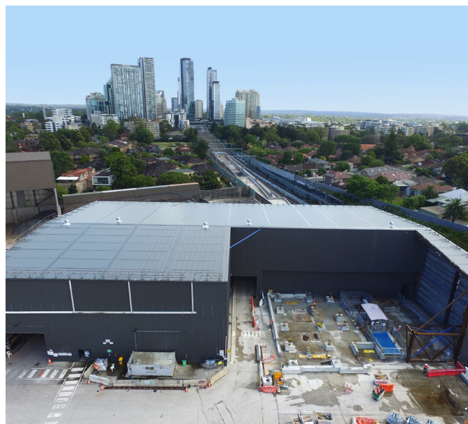
A section of the large gantry crane shed site has been removed to make room for above-ground construction of the Northern Dive Building, directly above the tunnels below.
