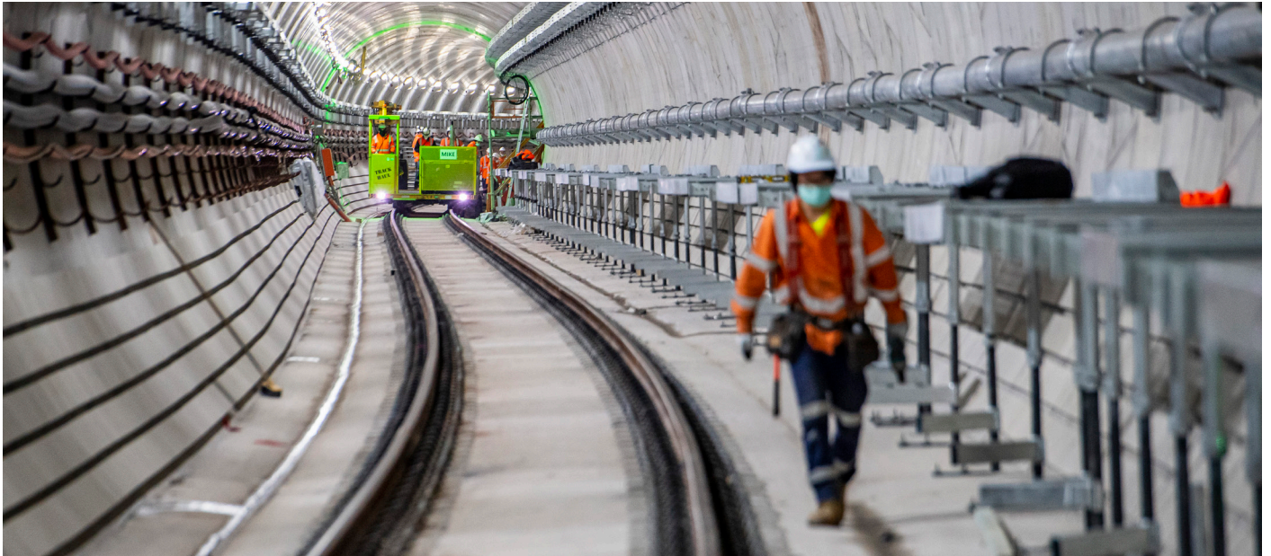
Work in the Sydney Metro City & Southwest tunnels between Chatswood and Crows Nest is now focussed on mechanical and electrical fit-out.
