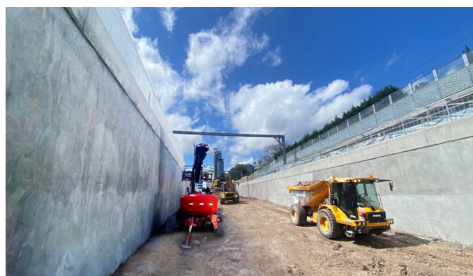
The ramps and track leading in and out of the tunnels at Chatswood are taking shape, with the base slab, track and overhead wiring to be installed during the first half of 2022.
