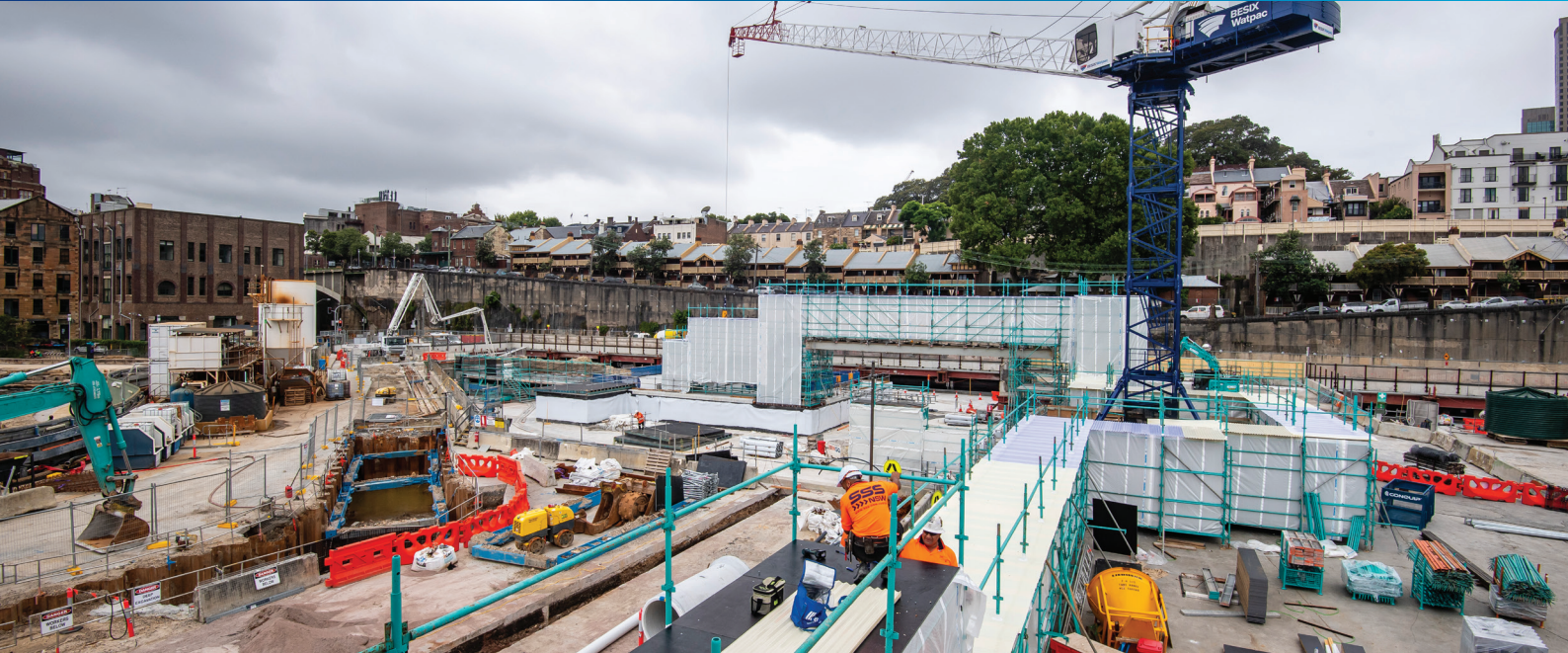
Construction taking place at the surface of the Barangaroo metro station site
