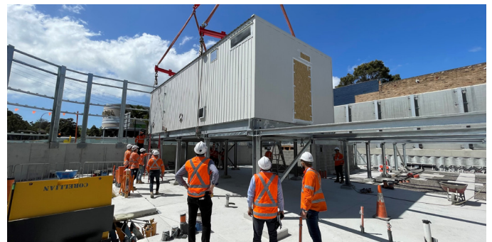
The Telecom Equipment Room being bolted into position by Kia Arbabi and the team.
