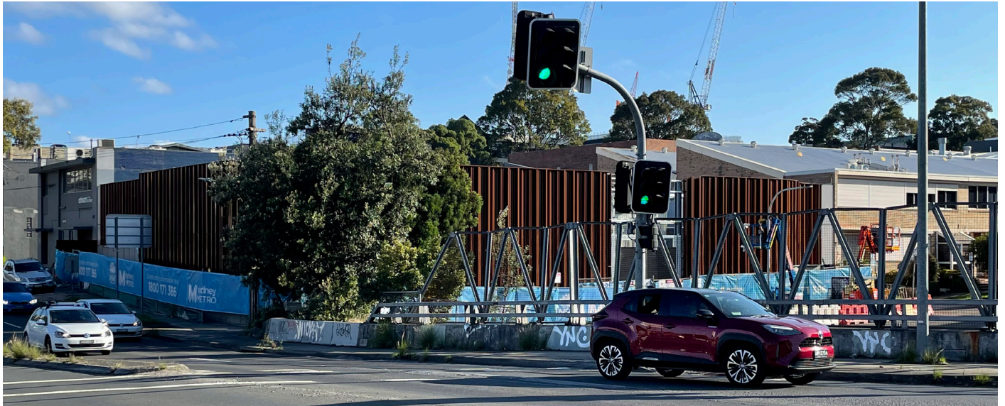
The Artarmon Traction Substation, at the corner of Reserve Road and Whiting Street, is nearing construction completion.
