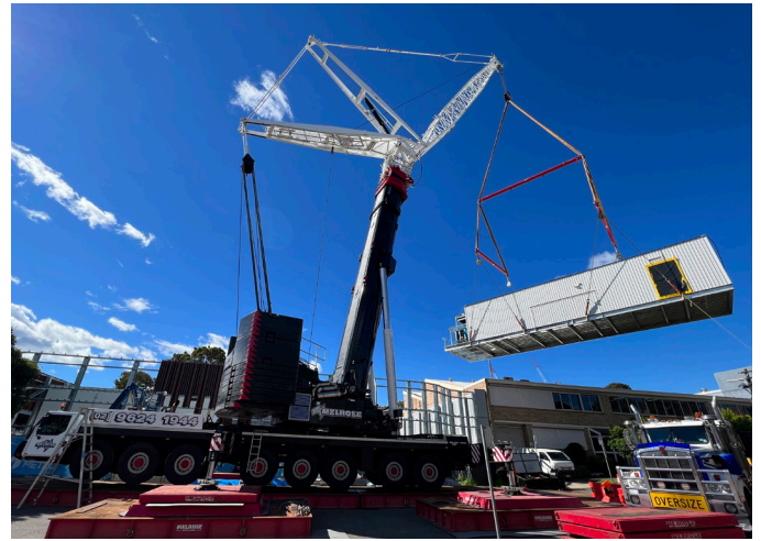
The last of the equipment rooms was lowered into place using a 500 tonne crane.
