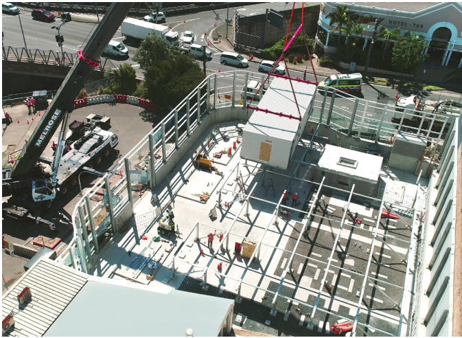
The Artarmon substation buildings were prefabricated in a factory before being craned into position on a supporting metal frame.
