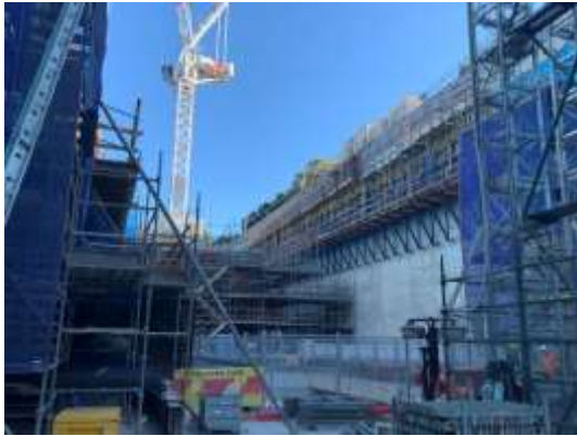
Station Box - Steelwork, formwork and wall pours through Level B3 and up
