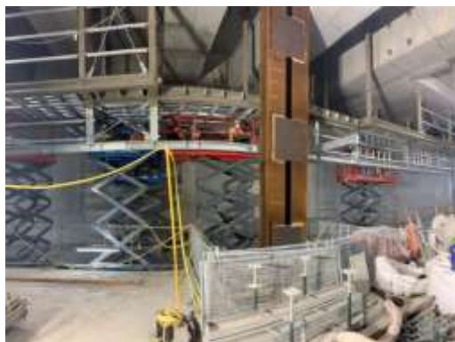
Over Track Exhaust (OTE) structural steel install, fireproofing spray and CFC sheeting
