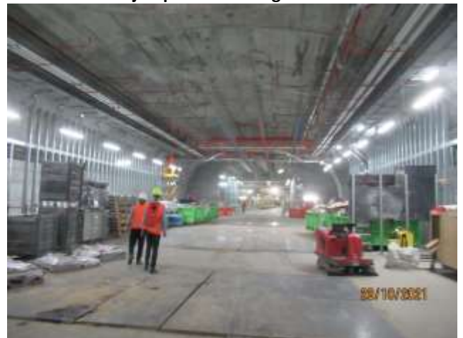
Pedestrian access way at platform level between MPS and MPN – fit out activities
