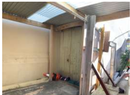
Preparations for use of Church Annex for Minor Ancillary Facility, with access constructed from existing site shed compound on south side. No fixings to church observed
