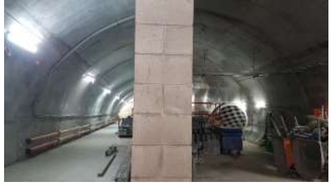
Eastern cavern back of house and OTE ventilation fans
