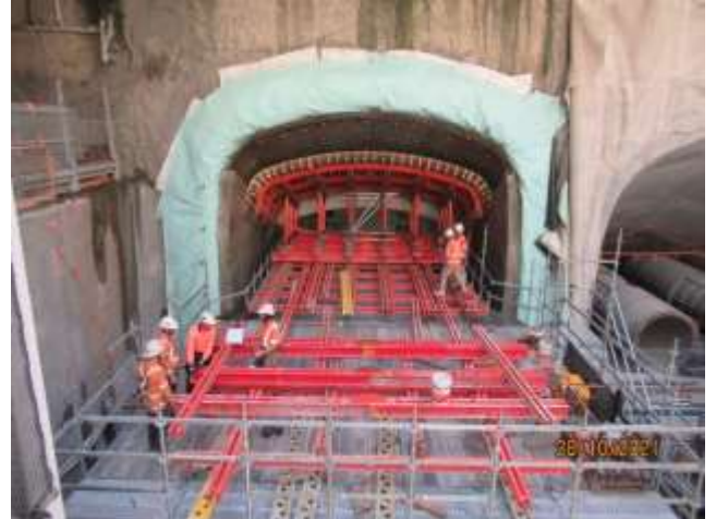
Last section of the access to the pedestrian tunnel between MPS and MPN
