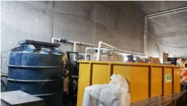
Pitt St North (PSN) water treatment plant
