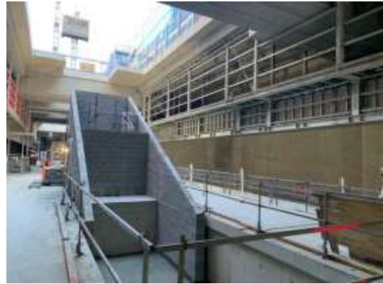
Levels B5 blockwork continuing for back of house and also for escalator void
