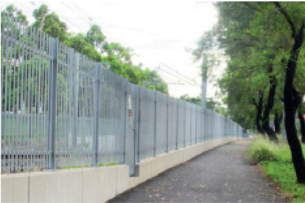
Homebush, Sydney. Rail corridor security fences should be robust, easily maintained, modular systems that are readily integrated with other urban design elements such as retaining walls.
