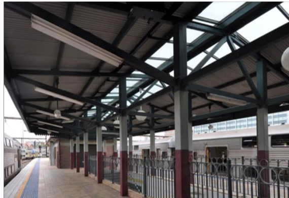
Figure 3: Typical awning extension on the Sydney Terminal platforms and extant balustrading (Source: Rappoport, 2013).
