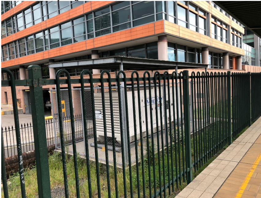
Photo 2: View from Platform 0 to the Transformer/substation at the southern extent of the site.
