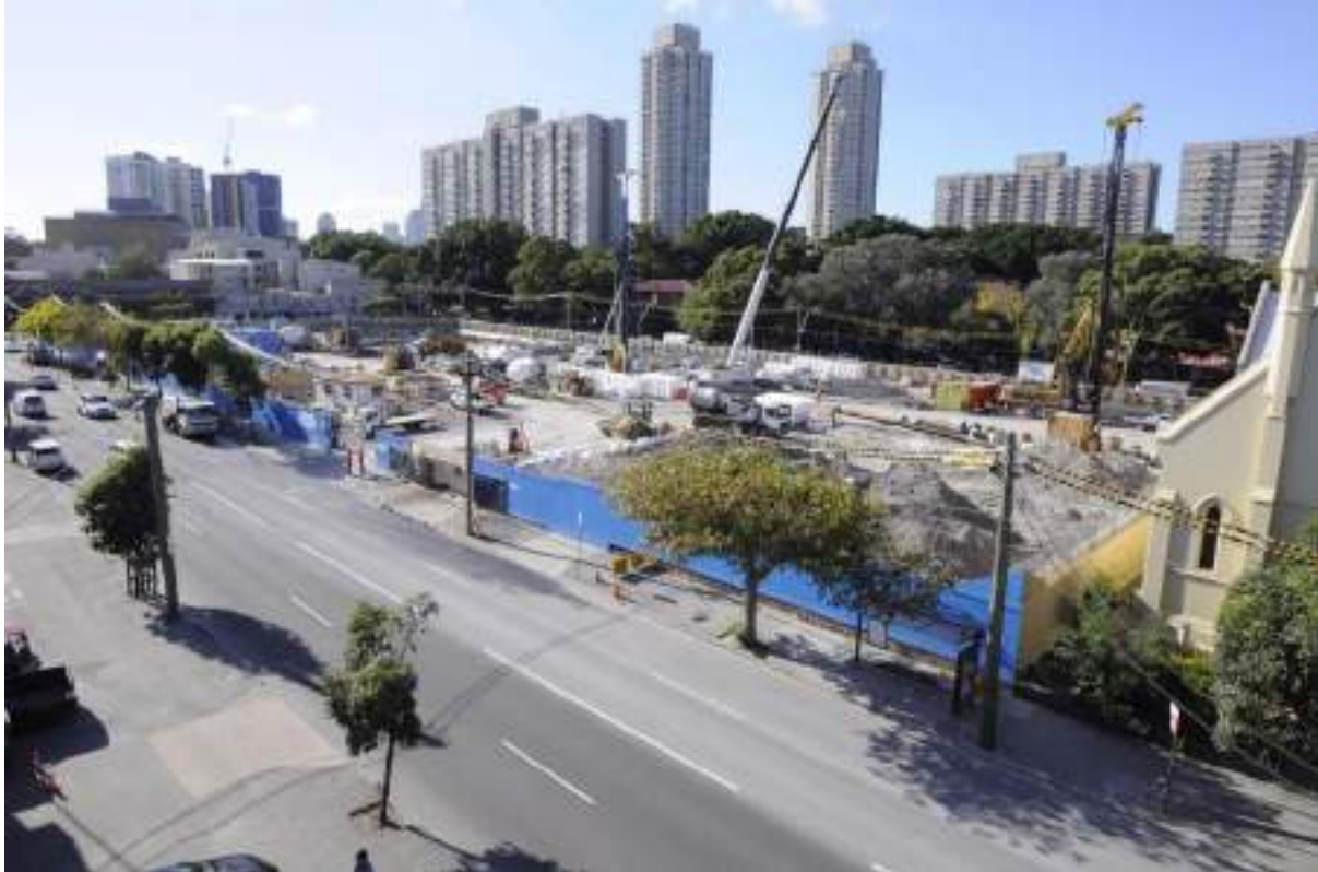
Figure 22 – The Site looking north-east along Botany Road (north of the Wellington Street intersection)
