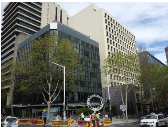
Figure 21: View of the subject site at the intersection of Miller and Berry Streets showing the commercial office building on the corner and the protruding blank side wall of the Victorian shop in 2016, prior to the commencement of demolition works. Source: OCP Architects, 2016
