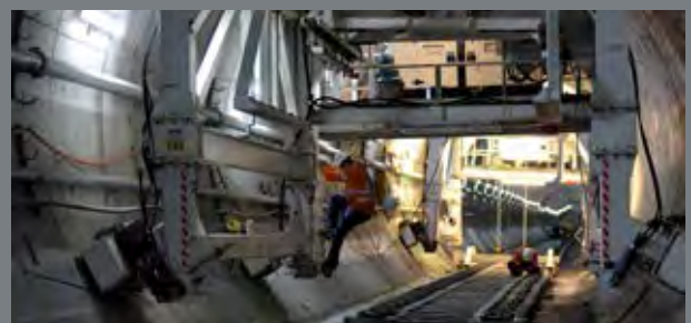
Fitting out the tunnels began in mid-2020, with the first tracks being laid in January 2021 at Chatswood.
