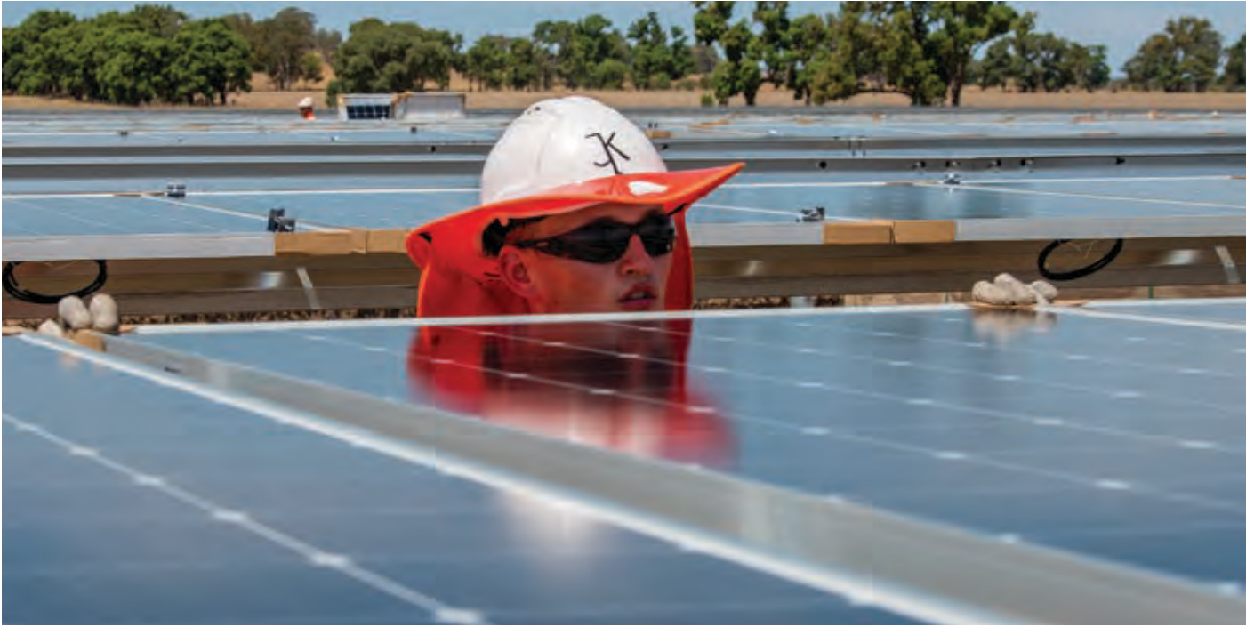
Beryl Solar Farm at Gulgong.
