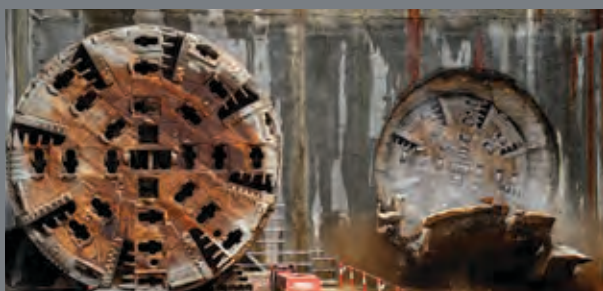
Tunnelling under the centre of Sydney finished in January 2020 when Mum Shirl, the last of four TBMs, arrived at Barangaroo.
