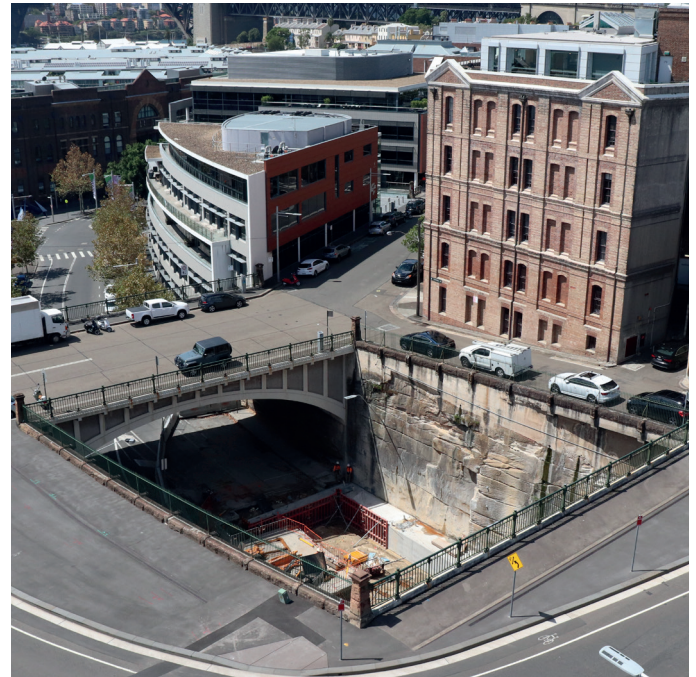
Location of the temporary access shaft on Hickson Road between Windmill Street and Dalgety Road
