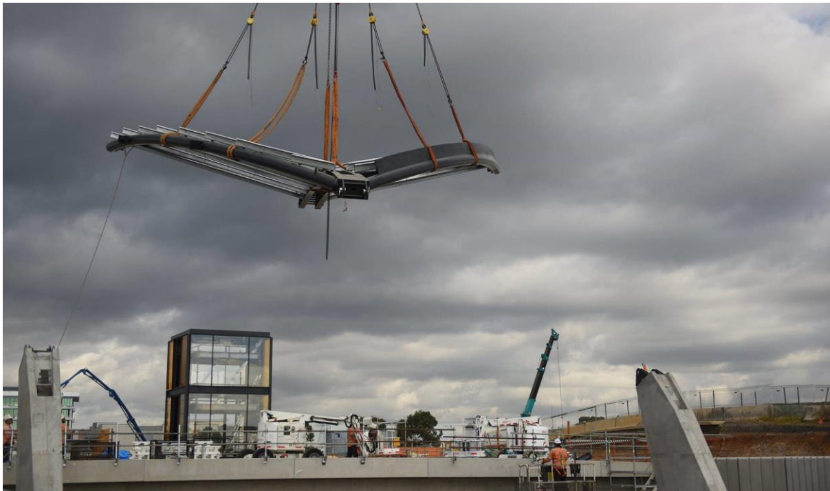
Figure 3 – Lift and installation of first section of a 100-tonne canopy at Bella Vista station
