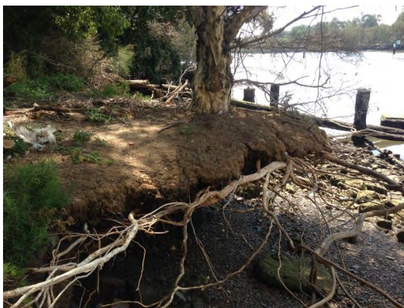
Plate 4.3: Undercutting and erosion of natural banks to the north of the wharf.
