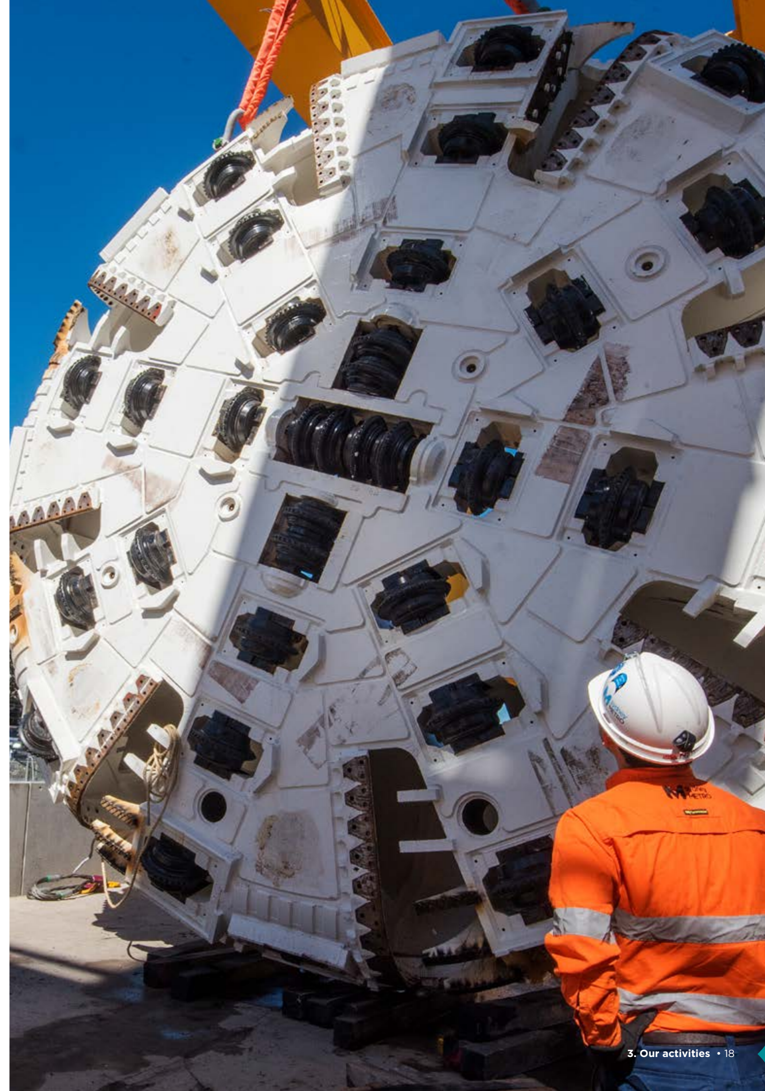
Right: The cutter head of tunnel boring machine Nancy being prepared for tunnelling at Marrickville.
