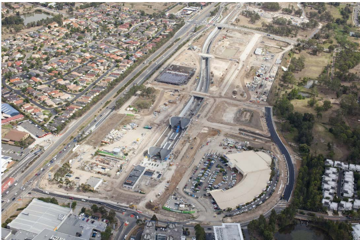
Figure 1-1 Aerial view of the construction of Sydney Metro Northwest Bella Vista Station (right), Old Windsor Road (Middle), Glenwood residential area – Swansea Court and Sharrock Avenue (left)
