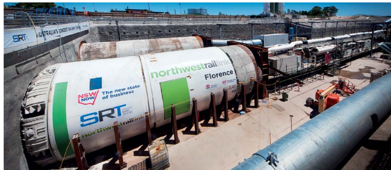
Florence was the second of four mega tunnel boring machines which tunnelled 30 kilometres on Sydney Metro Northwest
