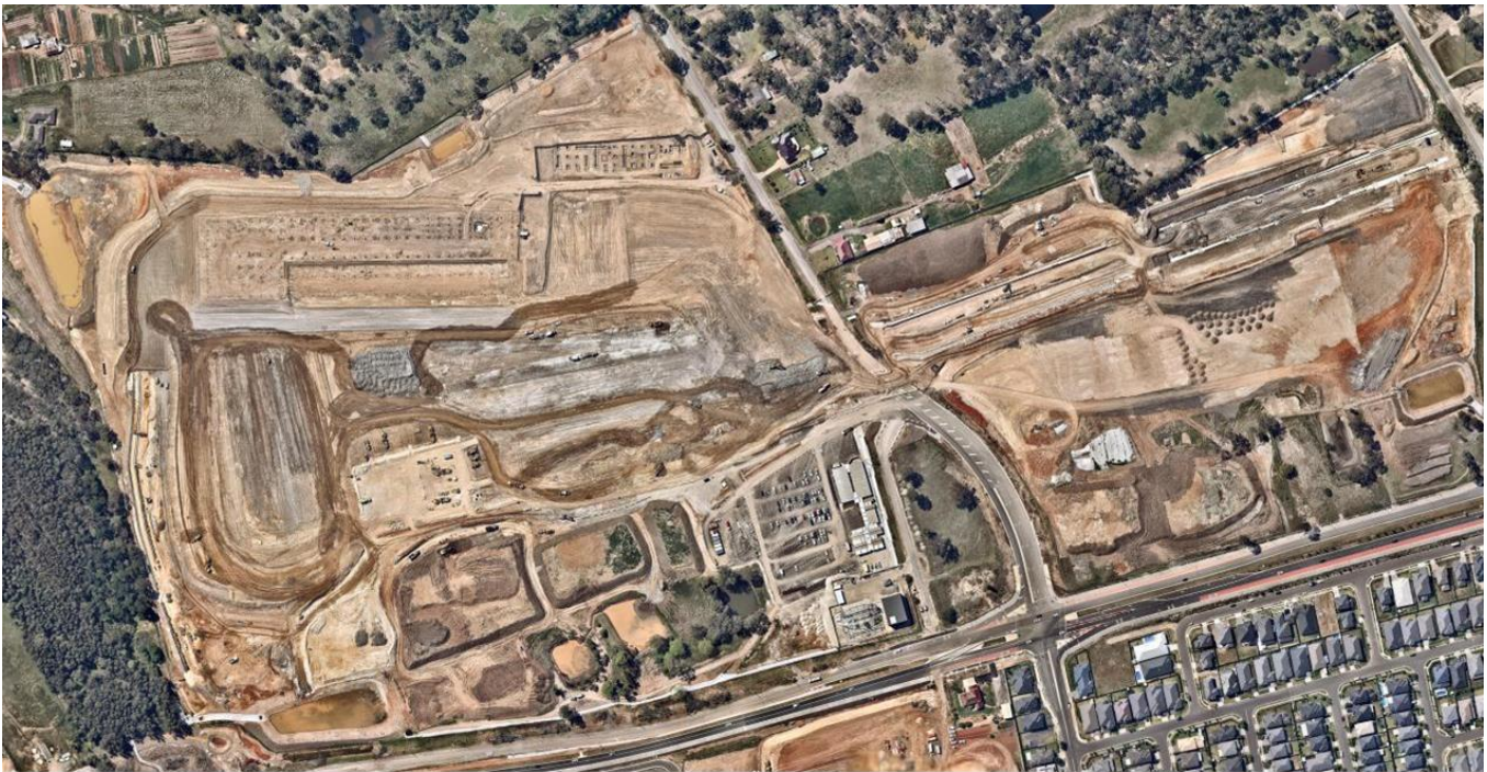
Figure 4 - Aerial Photograph of the SMTF and Cudgegong Road Station Sites on 15 Oct 2015
