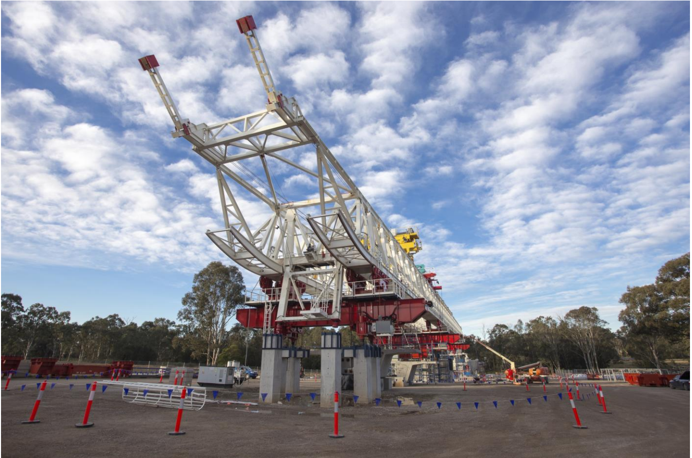
Figure 3 – Gantry Crane at the ISJV Kellyville Site
