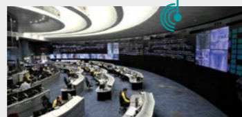
An example of a metro operations control centre
