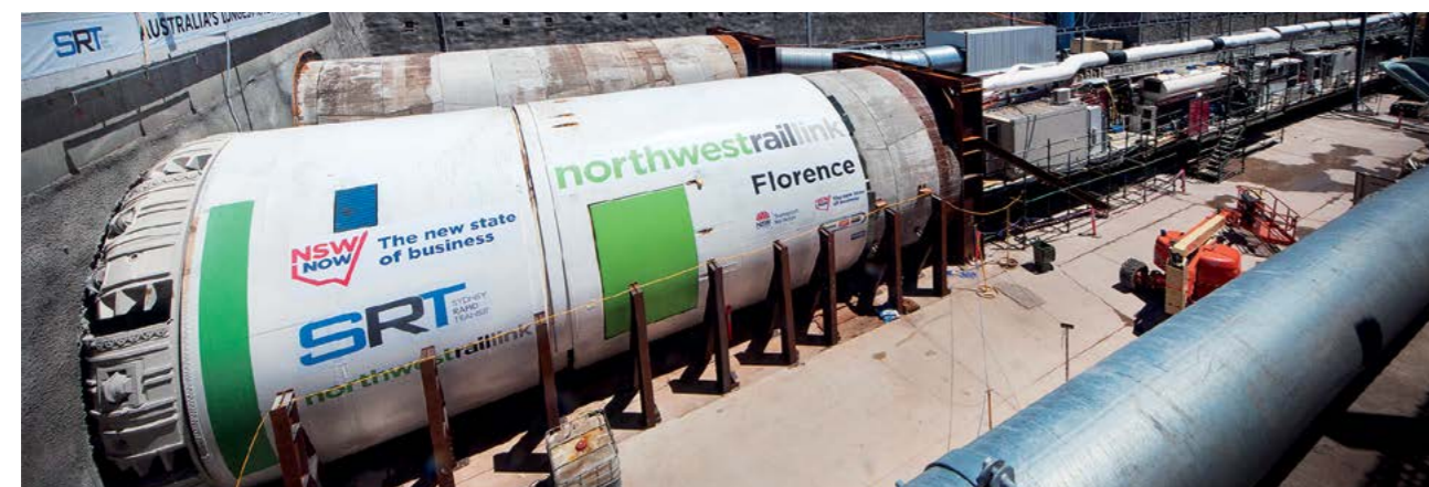
Florence was the second of four mega tunnel boring machines which tunnelled 30 kilometres on Sydney Metro Northwest
