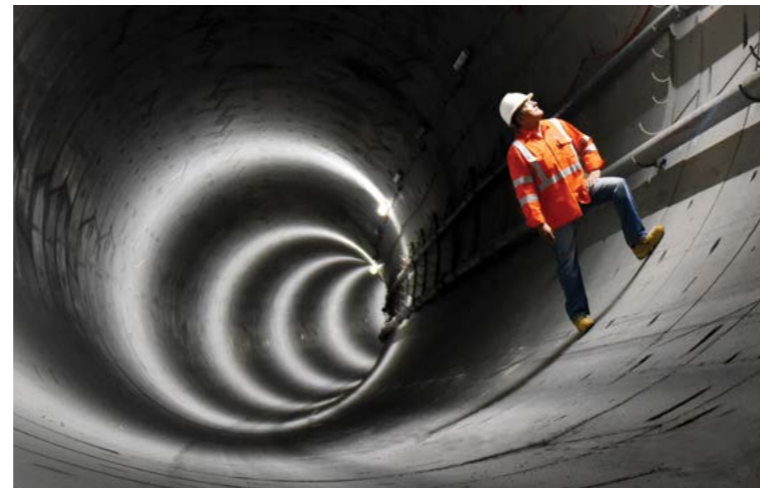
Australia's longest railway tunnels run 15 kilometres from Bella Vista to Epping on Sydney Metro Northwest
