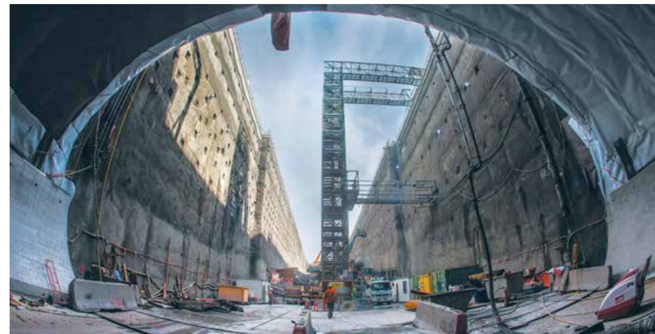
Looking out from the Castle Hill cavern into the station site, July 2015
