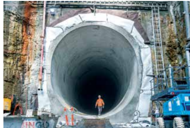
Two 300m long tunnels linking the new twin tunnels to the existing railway tunnels between Epping and Chatswood were completed in mid-2015
