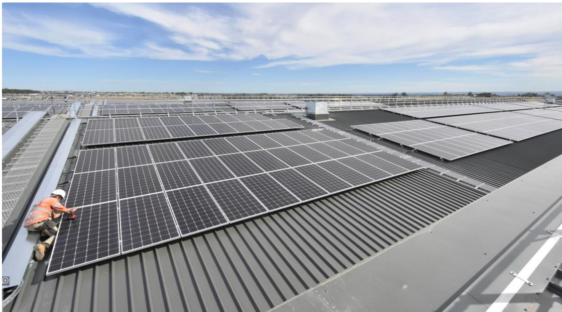
Figure 25 – 1.1 MW solar photovoltaic system being installed on the maintenance building of Sydney Metro Trains Facility.
