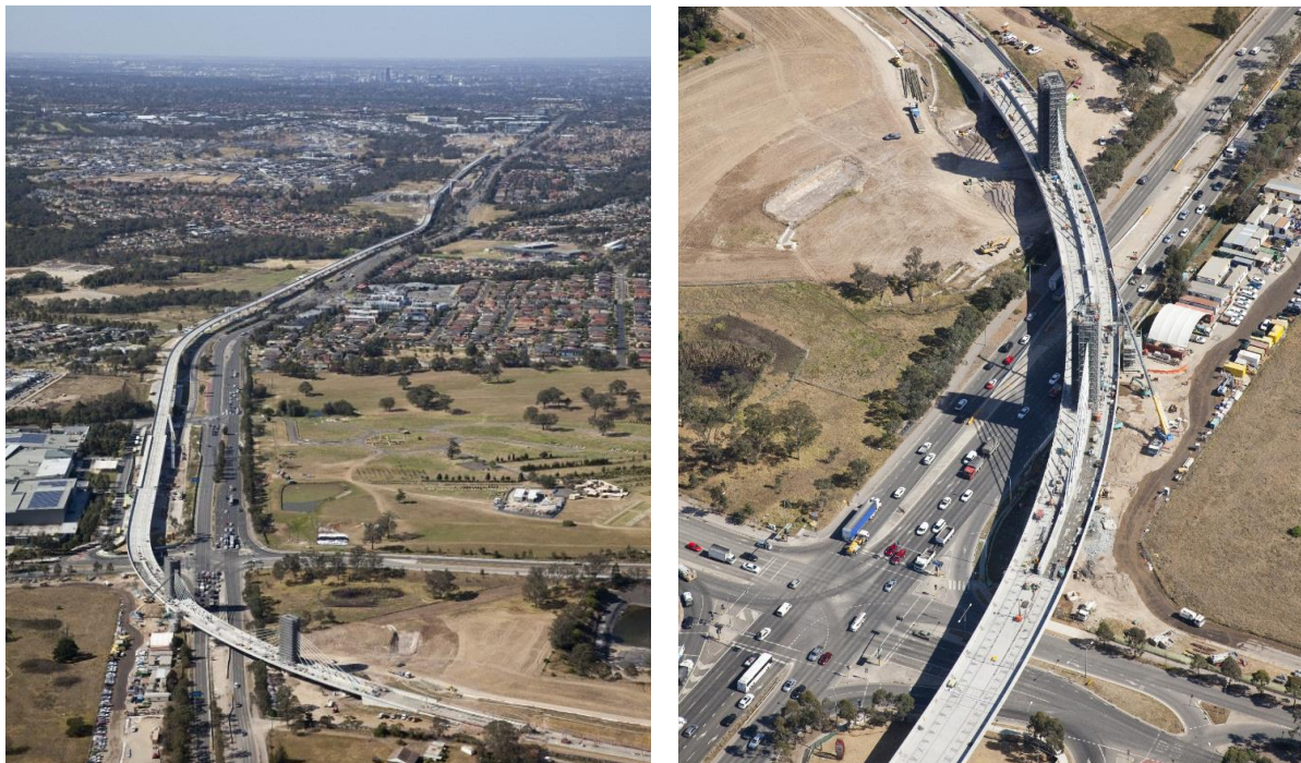
Figure 2 – Completed viaduct from Rouse Hill towards Norwest, and Windsor Road Bridge under construction. Images were taken in September.
