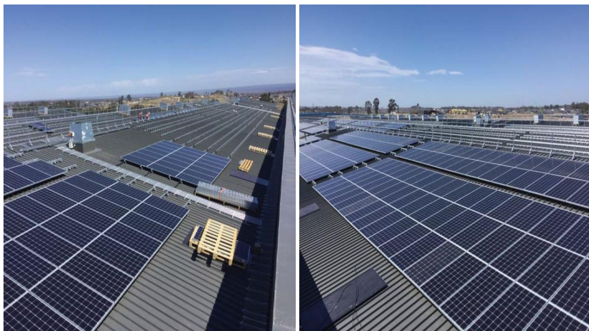
Figure 19 – 1.1 MW solar photovoltaic system being installed on the north-facing maintenance building rooftop
