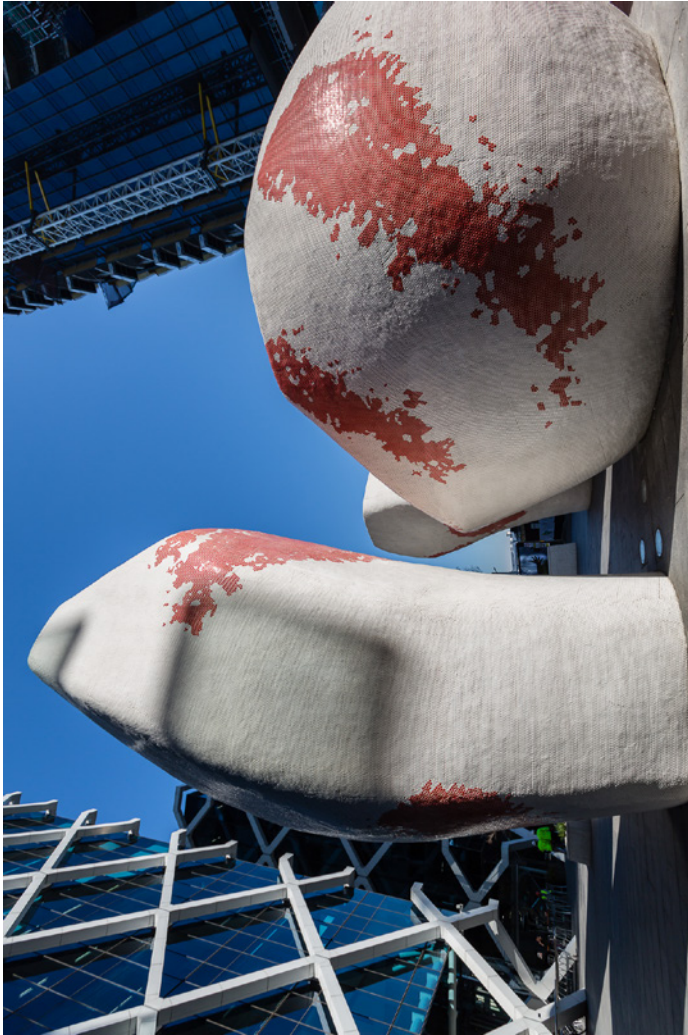
Sculptural plant extraction vents at One Shelley Street, Sydney. Artist: Anton James Source: TN SW
