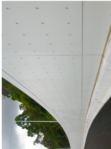
Gore Hill Freeway, Sydney. Provide retaining walls that are topped out by a consistent concrete capping beam. Source: AECOM.
