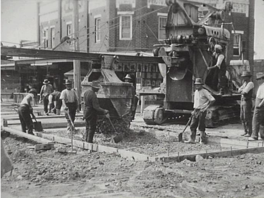
Figure 6-15: Lakemba c.1932, concreting Haldon Street. Source: Bankstown Library Collection via Pictorial Canterbury, item 020201.
