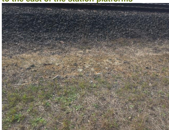
Plate 3: Marrickville Station survey unit-small area of erosion observed within the rail corridor to the east of the station platforms
