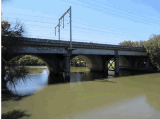
Figure 203: View of Canterbury (Cooks River) Underbridge - Main Line, north-east aspect (Sydney trains)
