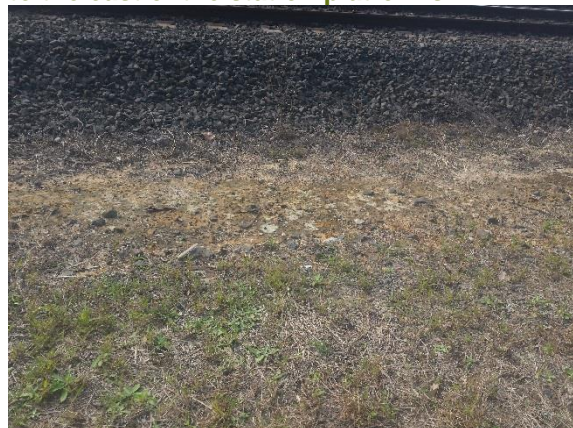
Plate 3: Marrickville Station survey unit-small area of erosion observed within the rail corridor to the east of the station platforms
