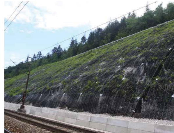
Combination of engineered slopes and low retaining walls to achieve a sculpted land form. Source: COX/HASSELL
