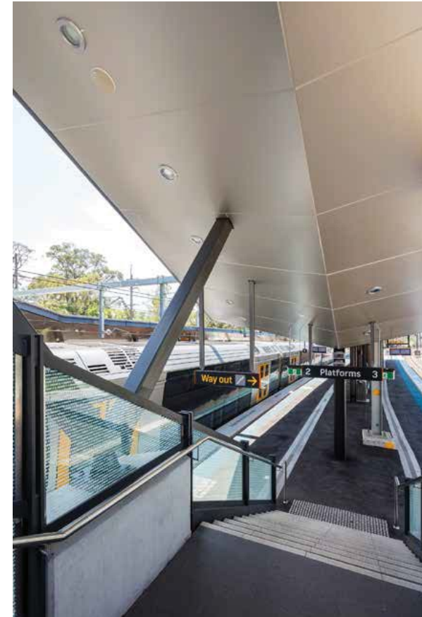
Engineered systems integrated into the platform canopy, Cheltenham Station Source: COX
