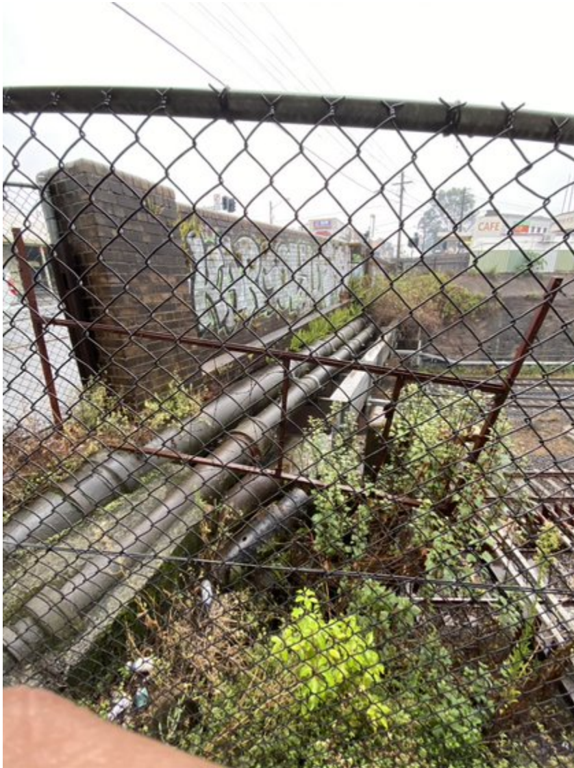
Figure 3: Canterbury Overbridge eastern side facing north, with both pipes, SJJ beam and vegetation surrounding pipes, proposed for removal within view
