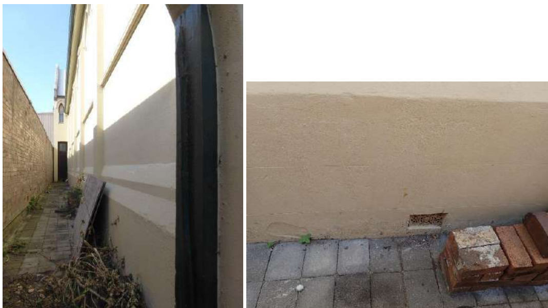
Figure 4 View along the passage on the north side (left), and the damp proof course will be immediately above the wall vent (right).
