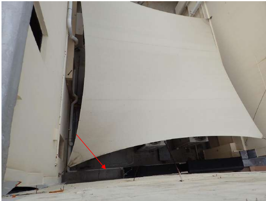
Figure 5 View into a lightwell behind the parapet wall at the top of the building. Option 2 is to locate the monitoring equipment on the upstand wall as arrowed.
