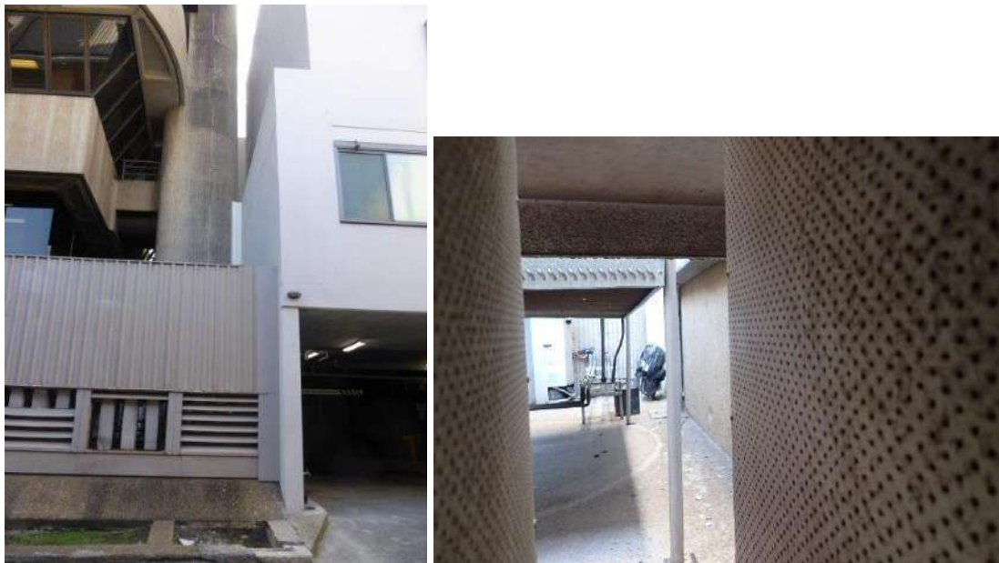
Figure 4 View of the boundary wall and screen to the air handling/air conditioning area on Clarke Lane (left), and view through the steel louvres to the space behind (right).
