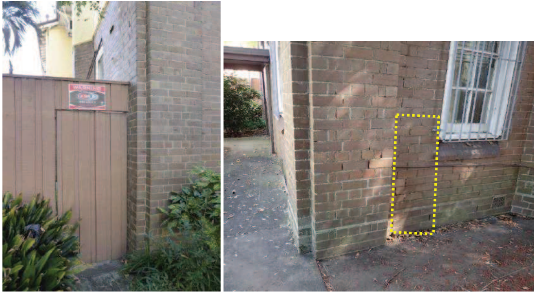
Figure 4 Views of the south-west (left) and south-east corners of Mowbray House. The vibration monitoring equipment will be located on the west wall behind the fence in the location as indicated on the east wall.
