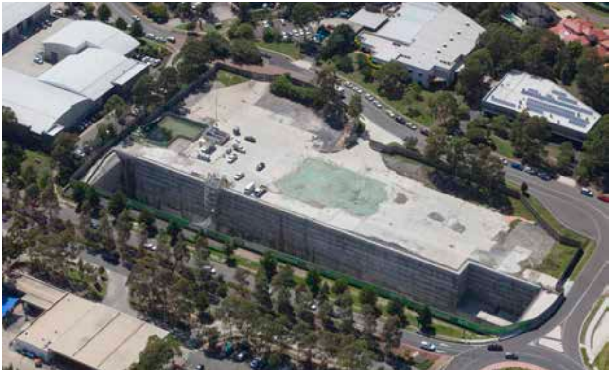
Figure 7: As it was in January 2016 – showing the Norwest construction site at the intersection of Norwest Boulevard and Brookhollow Avenue.
