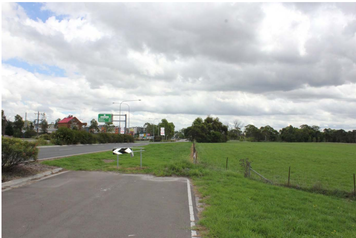
Photograph 3.1 Old Windsor Road to White Hart Drive construction area facing north. The Caddies Creek alignment of the road has been removed to the north of the road sign.
