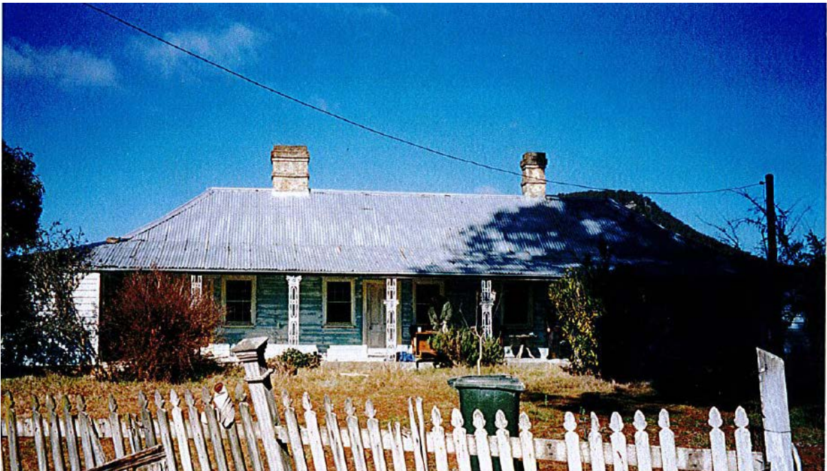
Photograph 3.2 Collit's Inn in 2001 prior to restoration works. (Source: Christine and Russell Stewart 2002, Section 4).
