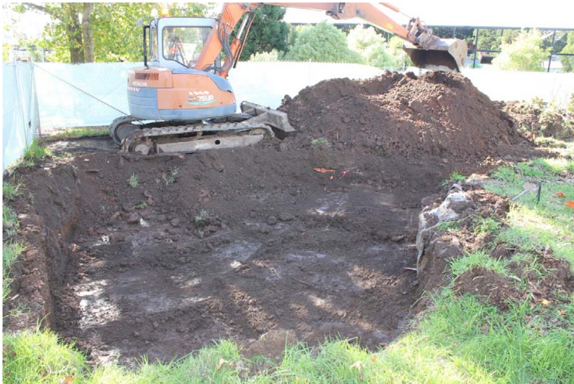
Photograph 3.6 Earthworks for the translocation of the Memorial Plane Tree located within the central portion of the reserve (facing west)
