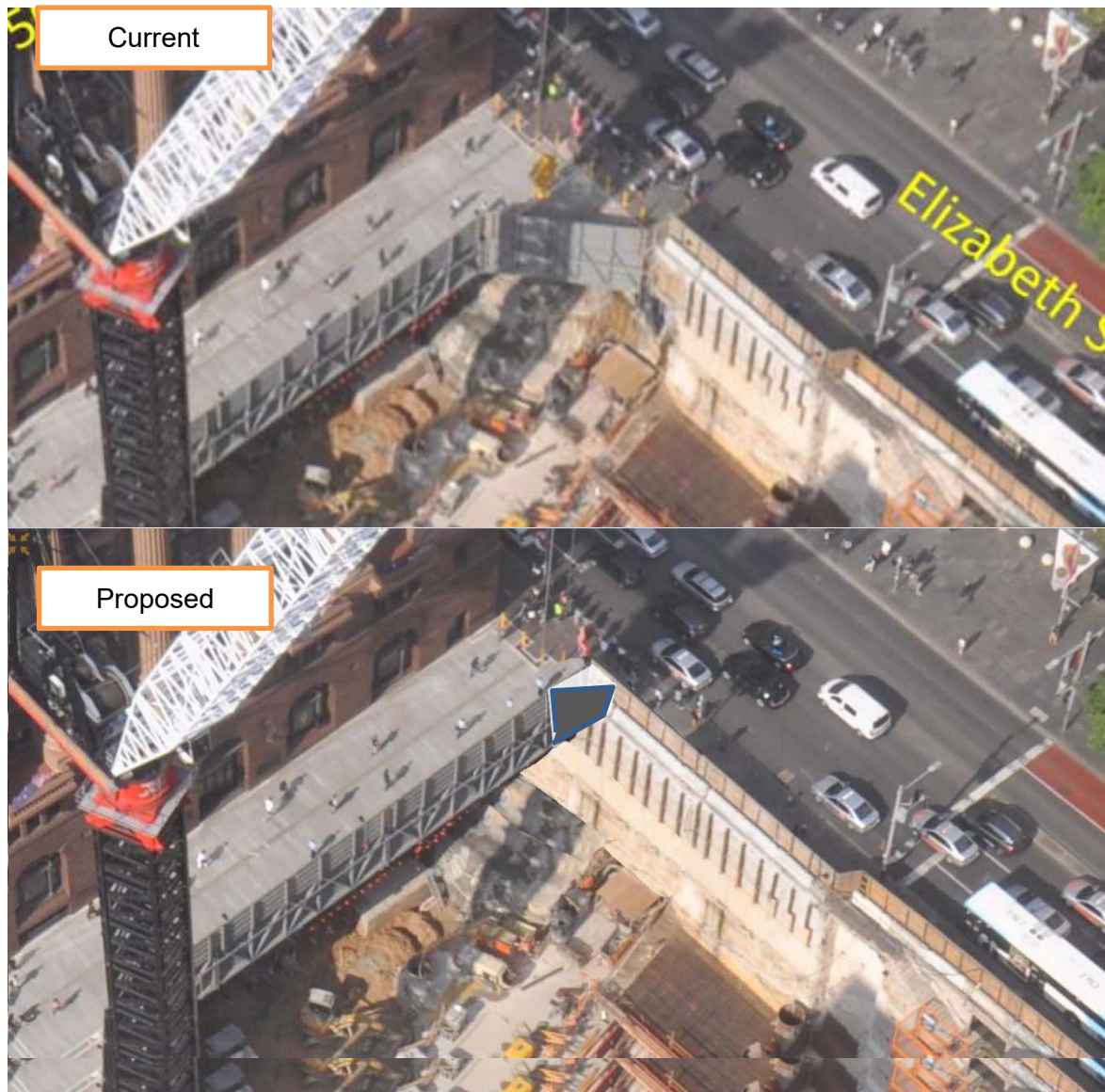
Figure 10: Current site photo of existing hoarding and artist's impression of completed works
