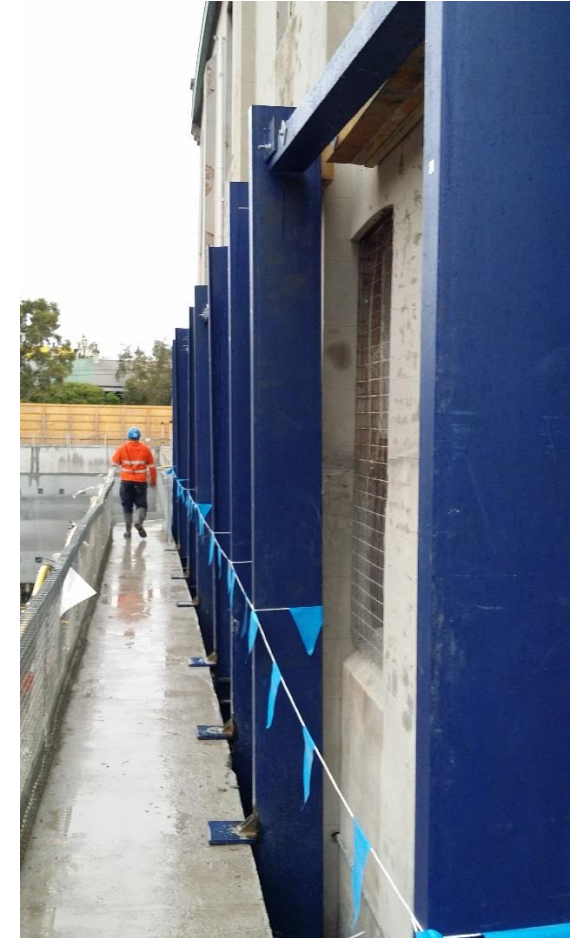
Right (alongside): Steel framework (in blue) as mitigation measure to prevent movement of the Waterloo Church Annex towards the Station Box excavation works (concrete capping beam atop piling, as shown).
