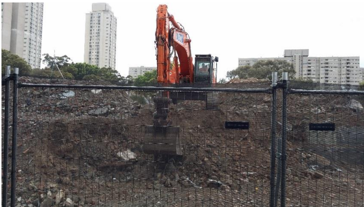
Excavator not fitted with quacker (non-tonal alarm), view from Cope Street.
