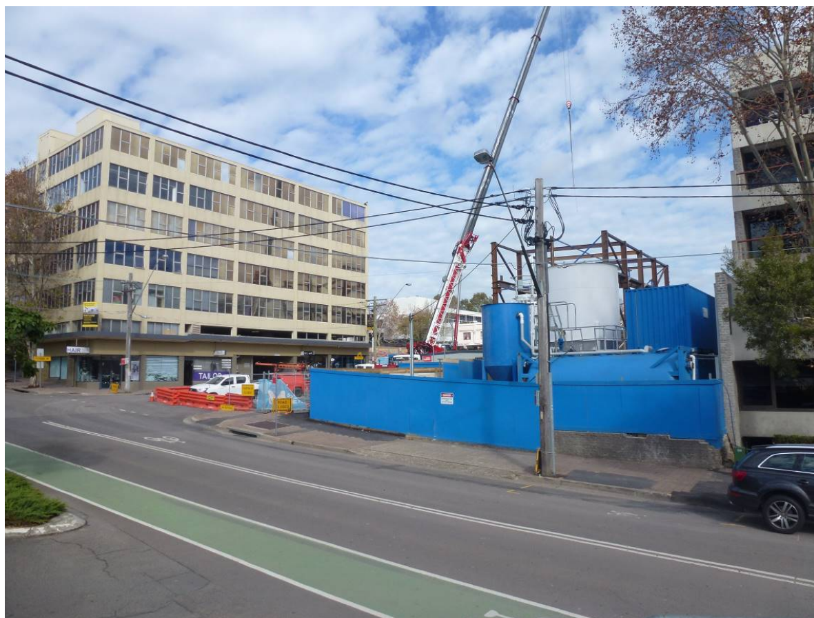
Figure 9 – Status of CSSI approval works on site C as of early June 2018
