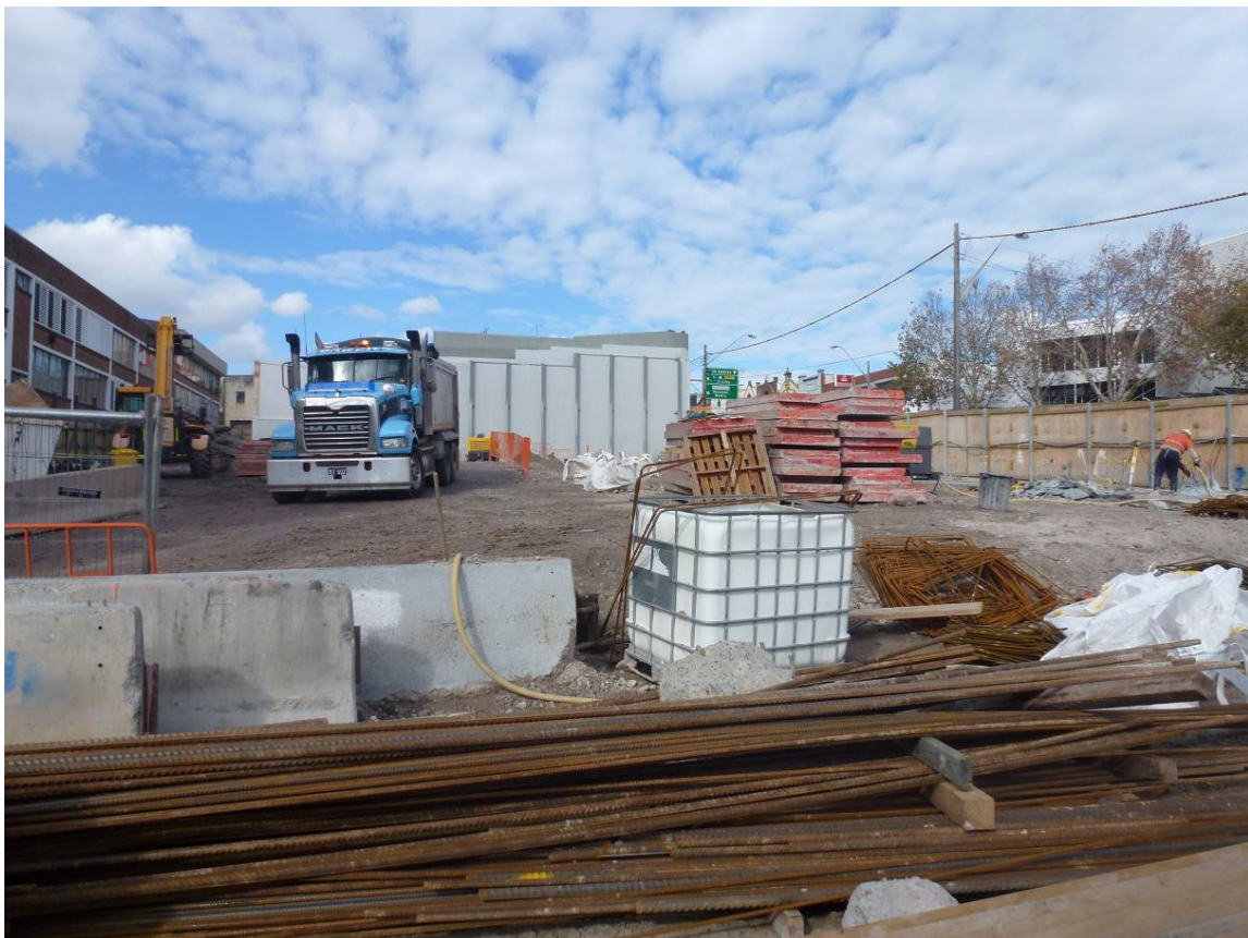
Figure 8 – Status of CSSI approved works on Site B as of early June 2018
